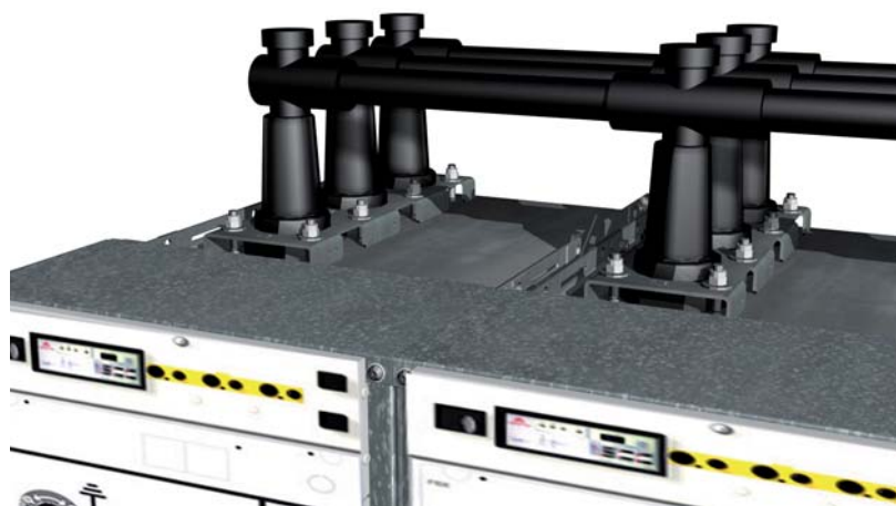
View of the busbars
