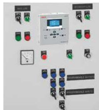
Control panel of a supply inverter with automation control unit Cat. N° 4226 80
