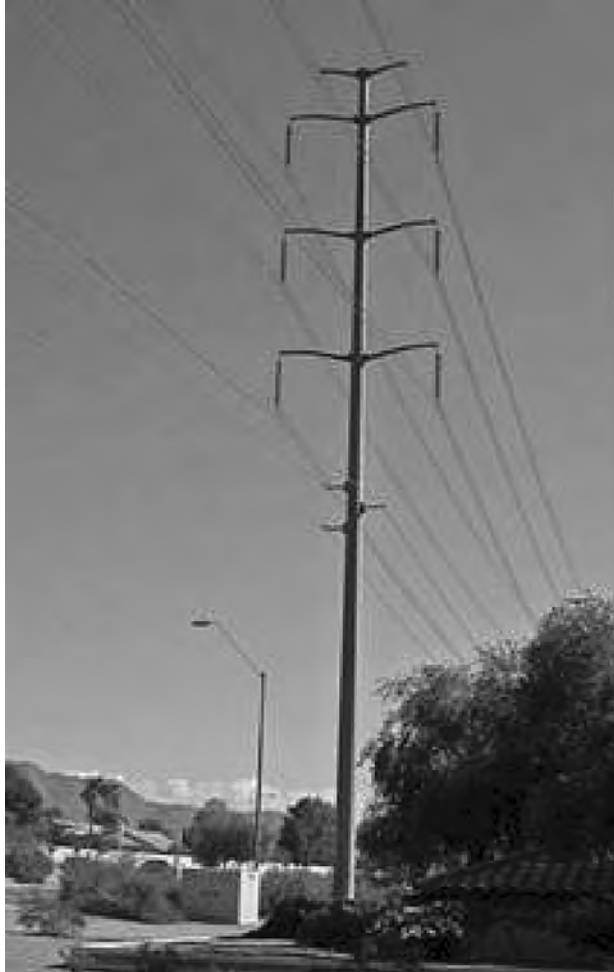
FIGURE 19.4 A 220 kV suspension tower.
