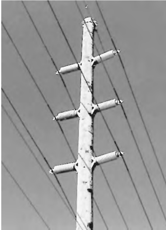
FIGURE 10.2 69-kV transmission line with post insulators.
