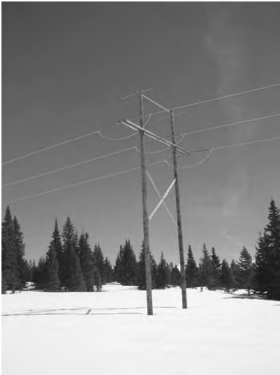
FIGURE 19.1 220 kV line with H-frame wooden towers.
