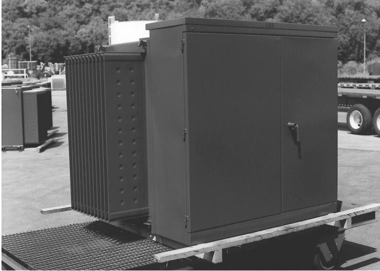
FIGURE 3.2 Typical three-phase pad-mounted distribution transformer. (By permission of ABB Inc., Jefferson City, MO.)
