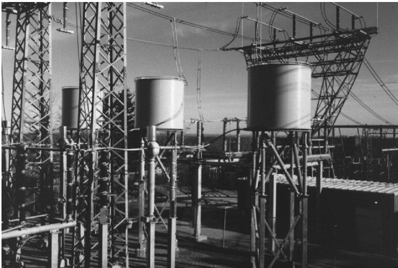
FIGURE 10.6 345 kV phase reactors.
