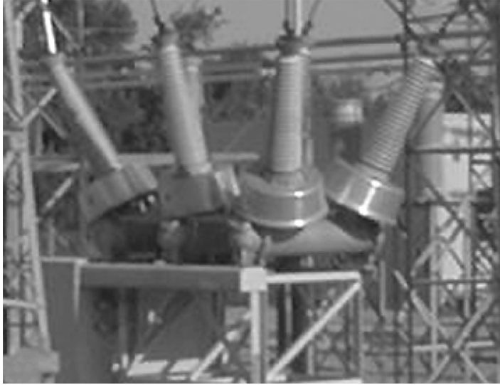
FIGURE 7.28 High-voltage circuit breaker with BCTs mounted underneath a metallic cover. (Photo courtesy of Kuhlman Electric Corp.)
