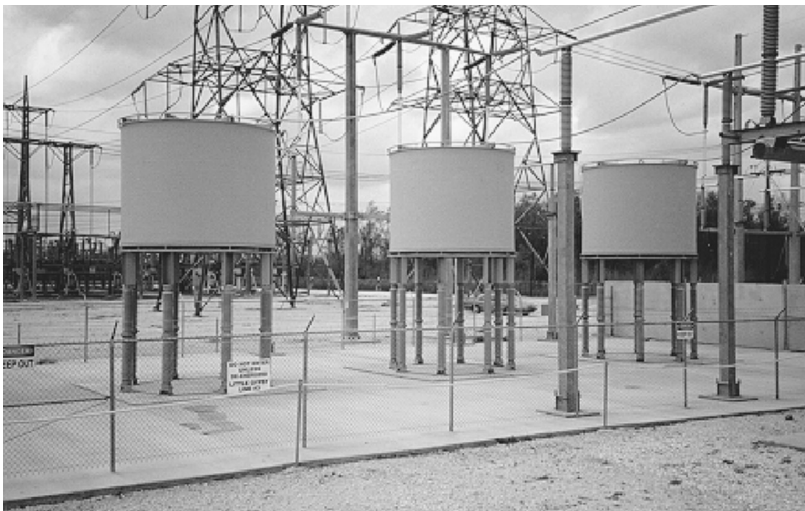
FIGURE 10.8 230 kV bus tie reactors.
