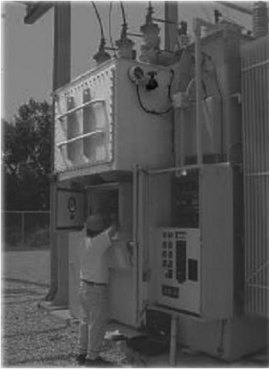
Externally mounted tap changer
