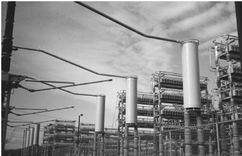
FIGURE 10.20 550 kV capacitor reactor.
