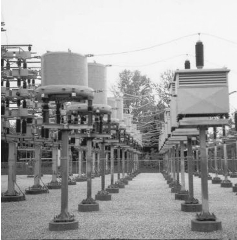
FIGURE 10.43 AC filter for an HVDC project; capacitors, tapped filter reactors, and separately mounted resistors.
