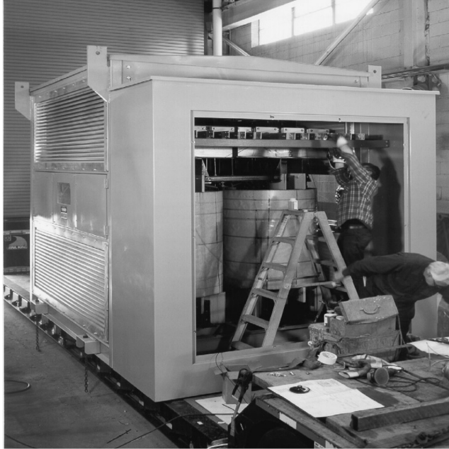
FIGURE 5.20 A 24-pulse dry-type transformer. 7000-kVA drive duty transformer, to be located in a tunnel, made of two 3500-kVA 12-pulse transformers. Each core and coil has 1100-V delta and wye secondary windings. Each core and coil has a 13,200-V extended-delta primary winding. One core and coil has its primary winding shifted -15^\circ , while the other core and coil has its primary winding shifted +15^\circ . One reconnectable primary spare core and coil can be used to replace either core and coil assembly. (Photo courtesy of Niagara Transformer Corp.)
