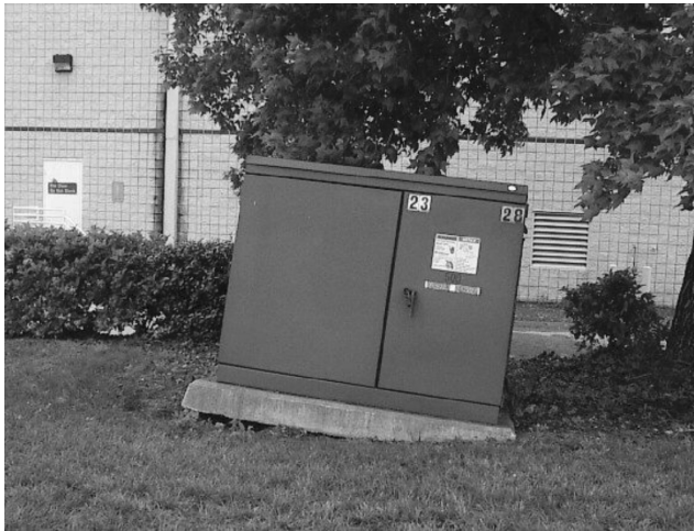
FIGURE 3.35 Tilting pad mount transformer.
