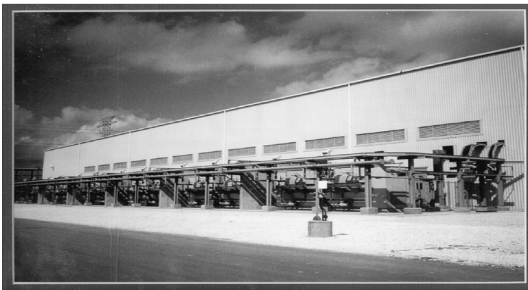
FIGURE 5.21 A 36-pulse system made up of 12 transformers with six types of six-pulse transformers for high-current electrochemical rectifier duty. Each transformer is 11,816-kVA ODFW with 426-V delta secondary windings. Each transformer has a 34,500-V primary with the shifts shown in Table 5.7 for a 36-pulse system. (Photo courtesy of Niagara Transformer Corp.)
