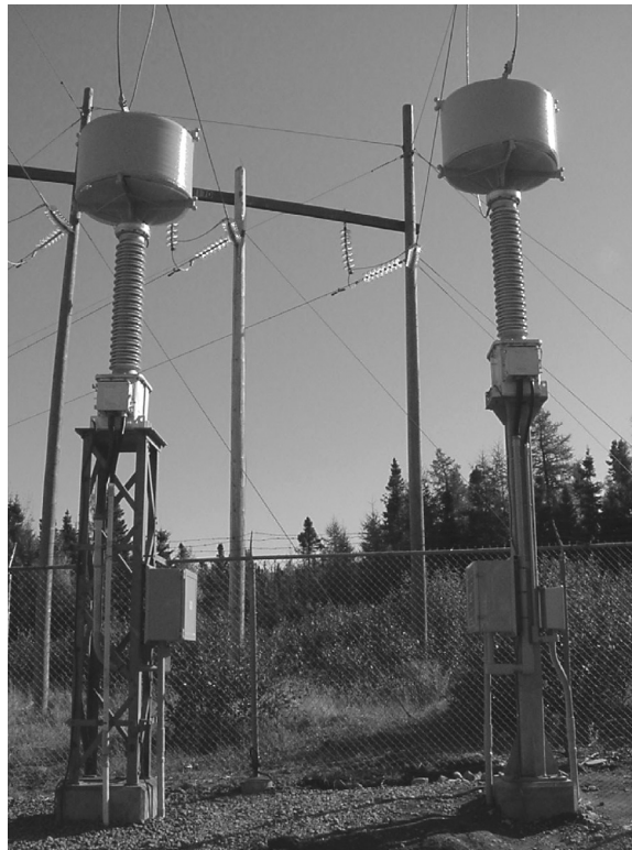
FIGURE 10.50 Line traps mounted on top of CCVTs.
