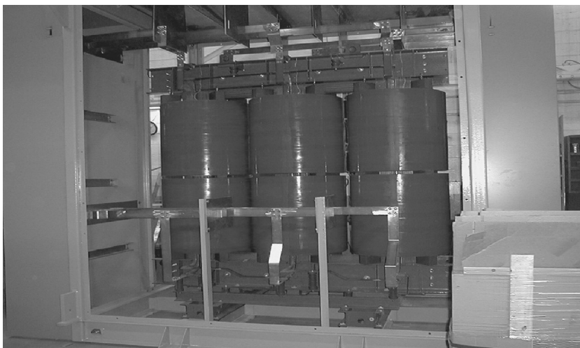
FIGURE 5.19 A 12-pulse Circuit 31 5450-kVA, 4160-V delta primary to 2080-V delta and wye secondaries, cast-coil transformer in case. (Photo courtesy of Niagara Transformer Corp.)
