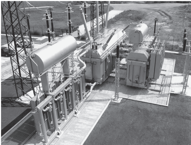
FIGURE 4.14 Quadrature booster set (300 MVA, 50 Hz, 400 \pm 12 \cdot 1.25\% / 115 \pm 12 \cdot 1.45^\circ kV). (By Courtesy of EVN Energieversorgung Niederösterreich Austria and Siemens AG, Germany.)
