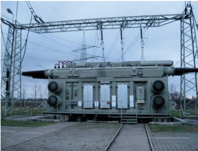
Figure 8.7 Overview of a transformer.
