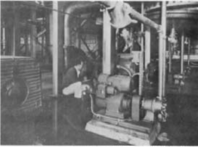
FIGURE 1 Pump application utilizing typical mechanical adjustable-speed belt drives (Reliance Electric)
