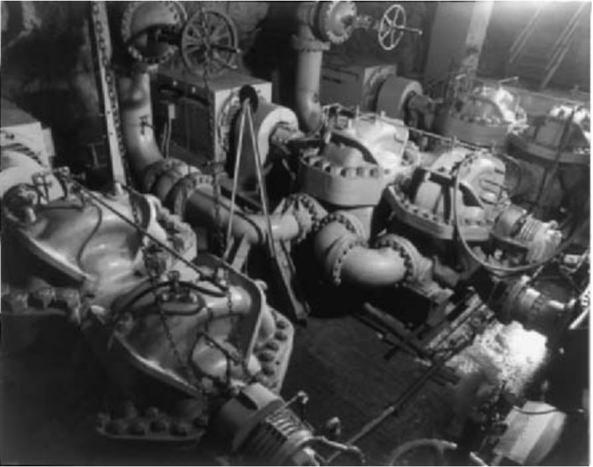
FIGURE 14 Three 2000 HP (1490 kW) pumps in one room in a zinc mine (Hazleton Pumps, Inc.)
