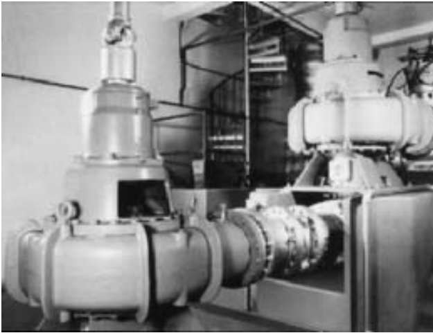
FIGURE 103 An installed vertical sewage pump similar to that shown in Figure 102 (Flowserve Corporation)
