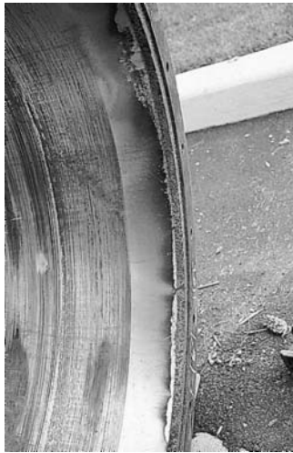
FIGURE 4 Galvanic corrosion is evident on this pump section. Note the high corrosion rate on the interior diameter of the carbon steel flange that is attached to the stainless steel shroud.
