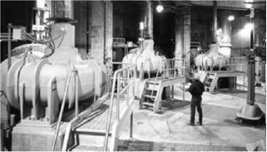
FIGURE 5 Vertical sewage pumping units at the South System Pump Station, Deer Island in Boston, MA containing (8) 36 in (915 mm), 46,300 gpm (10,510 m 3 /h) pumps driven by 1250 hp (932 kW) variable speed motors (FlowsERVE Corporation)
