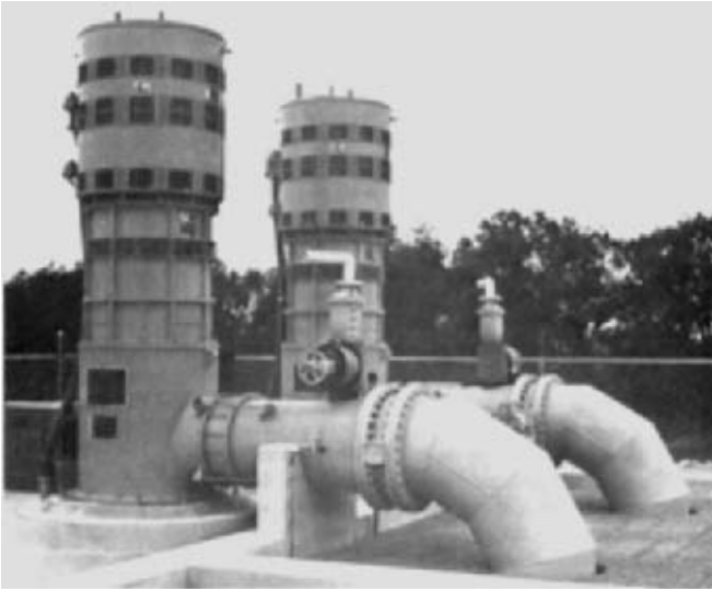
FIGURE 10 Raw water pumping station for North Texas Municipal Water District, showing vertical turbine pumps with variable-speed drives (Flowsolve Corporation)
