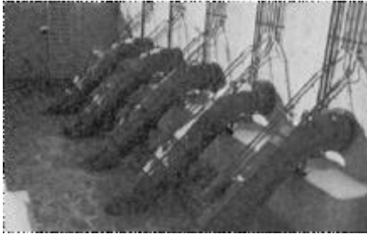
FIGURE 7 Five 42-in (107-cm) double-staged hydraulically driven water pumps with design flows automatically varying from 0 to 50,000 gpm (0 to 11,550 m 3 /h) (M & W Pump)
