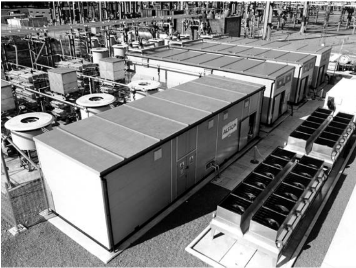
Figure 4.22 View of 225 MVA STATCOM
