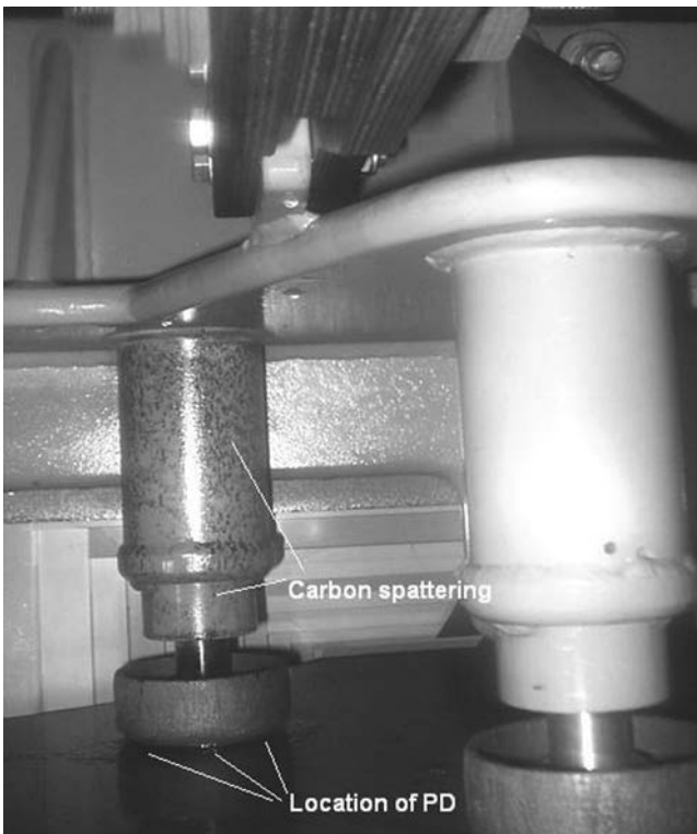
Figure 21.24 Transformer internal partial discharge from a core clamp
