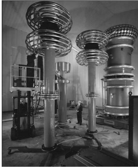
Figure 6.16 Resonant test system for 650 kV, 31 A AC
