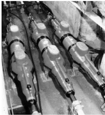
Figure 6.14 A joint bay showing joint protection boxes fitted to joints
