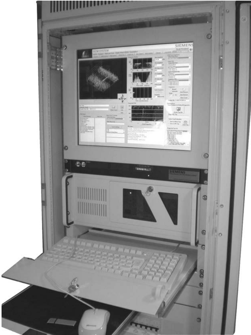
Figure 21.30 ISCM control cubicle showing PDM diagnostics display
