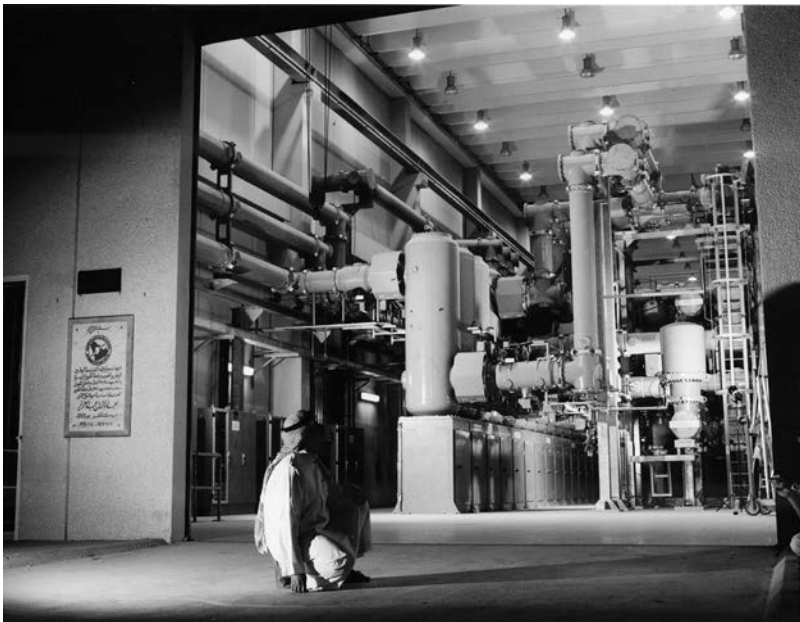
Figure 3.13 Example of 420 kV GIS equipment on a recent substation project in the Middle East (Courtesy VA Tech Reyrolle)
