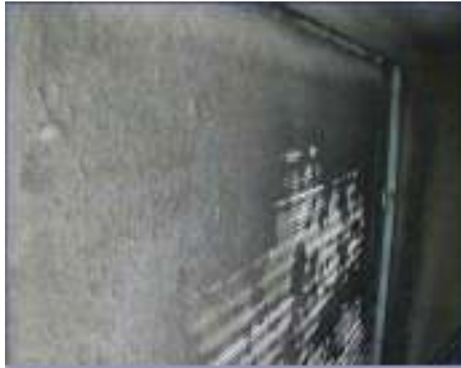
Figure 9.7.1. Cooling coil requiring cleaning
