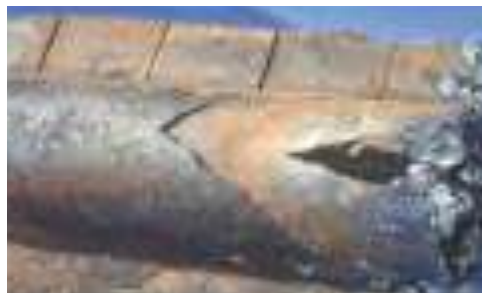
Figure 9.2.9. Boiler tube – failure (rupture)
