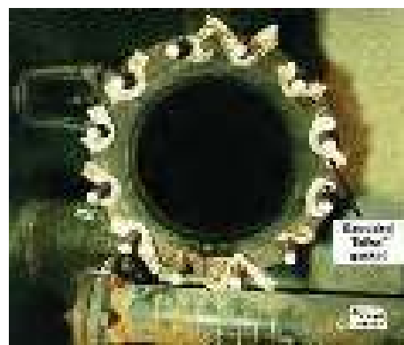
Figure 9.3.8. Failed gasket on blind flange
