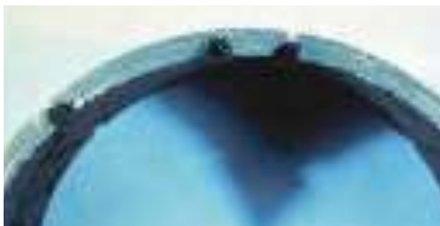
Figure 9.2.10. Feed-water pipe – oxygen pitting
