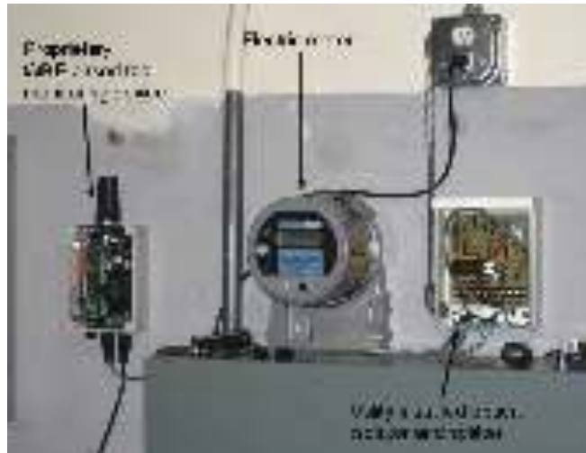
Figure 8.9.1. Installed wireless monitoring system for WBE-based system
