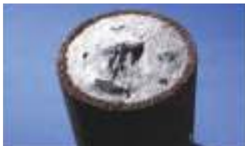
Figure 9.2.8. Boiler tube – scale deposit
