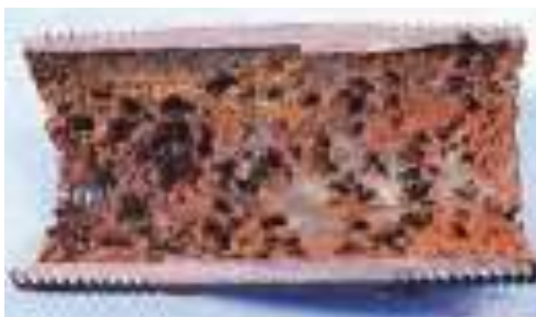
Figure 9.2.12. Condensate pipe – oxygen pitting
