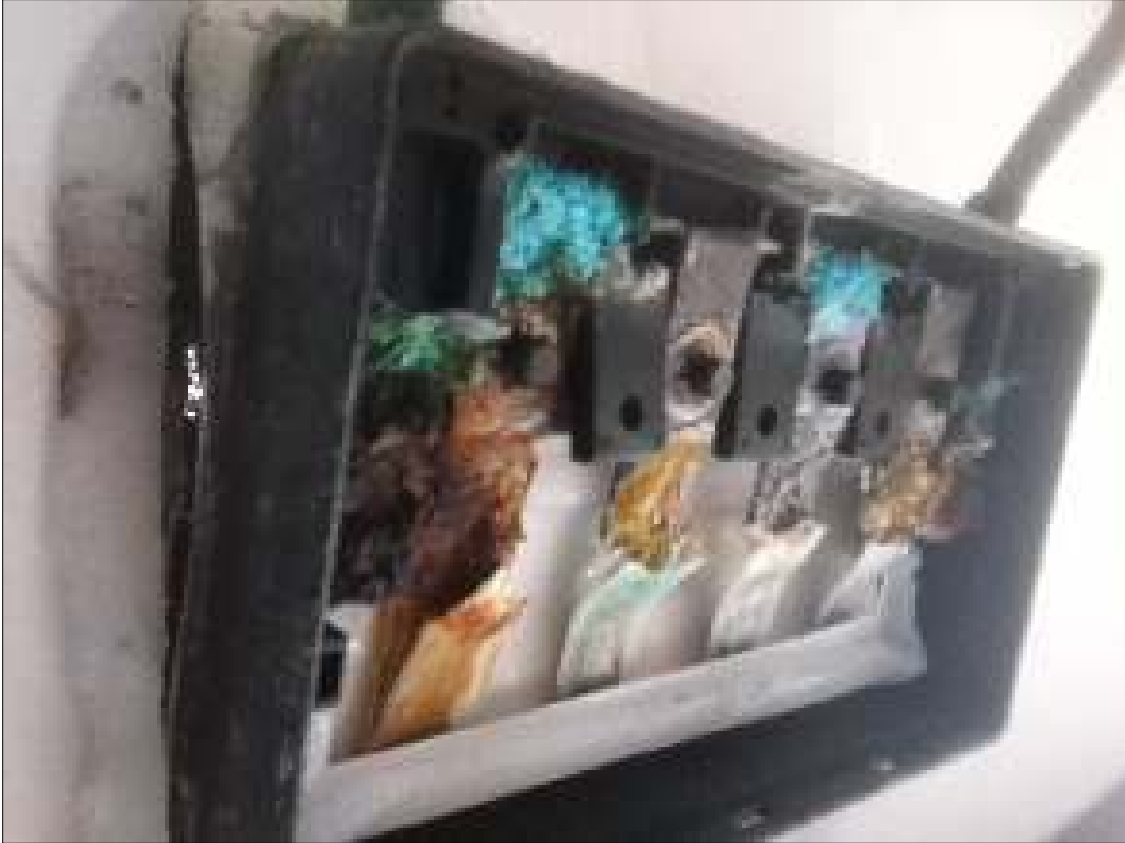
Figure 19. Manual inspection and testing requires opening NEMA-rated enclosures. The integrity of any enclosure seal must be restored after opening to avoid moisture damage as in this module junction box. Photo by Andy Walker, NREL
