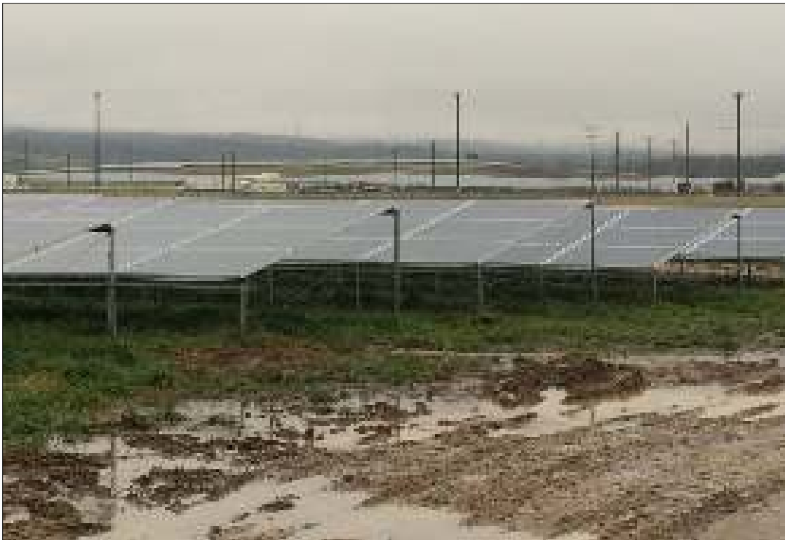
Figure 5. Drainage and storm-water run-off are difficult to improve after the PV array is installed, requiring diligence in design and construction of storm-water management systems. Photo by Andy Walker, NREL
