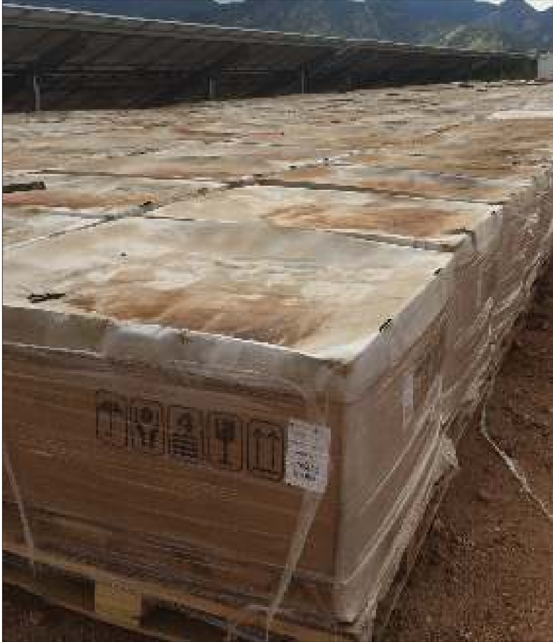
Figure 16. Failure to follow product box handling and storage requirements can cause damage when moved and void a warranty. The umbrella symbol on this box indicates it should be kept dry and the box might fail when picked up with a forklift. Photo by Andy Walker, NREL
