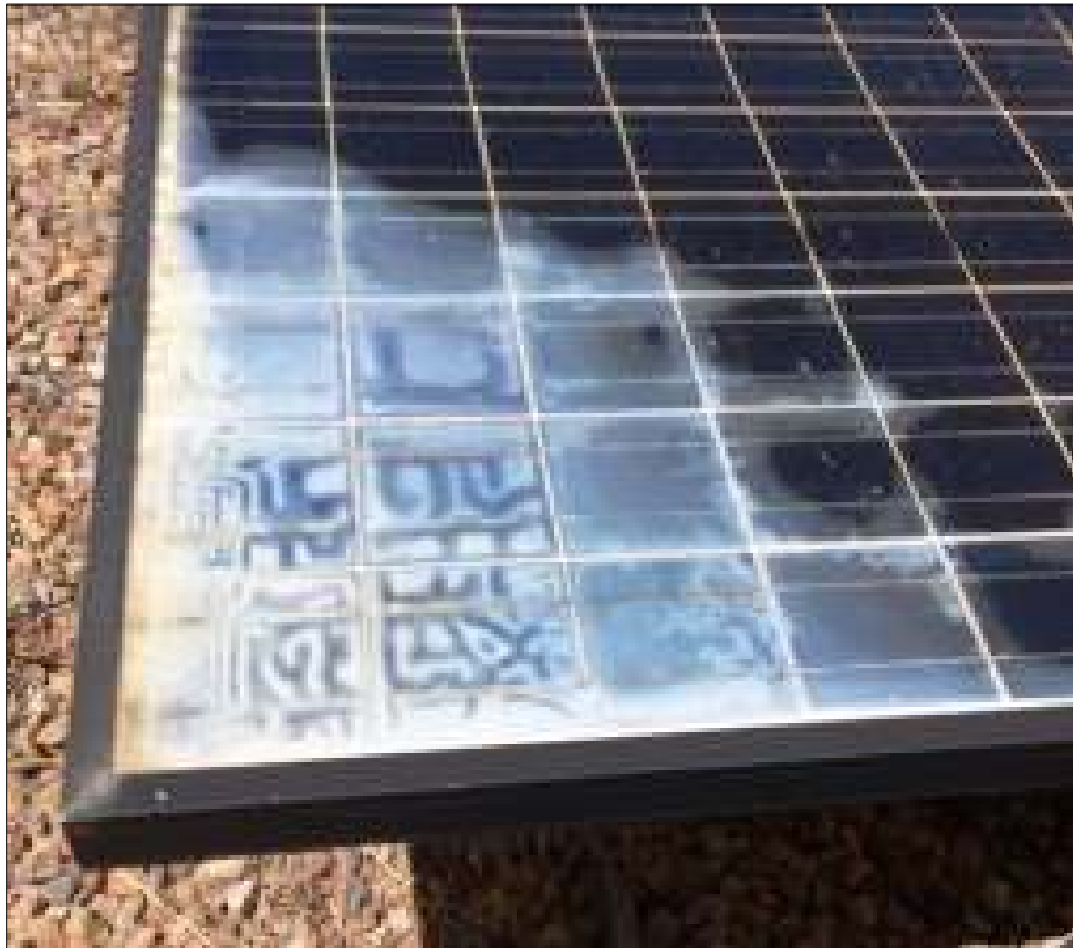
Figure 14. Failure in materials and workmanship, such as encapsulant of this module, are often covered by product manufacturer's warranty. Photo by Andy Walker, NREL
