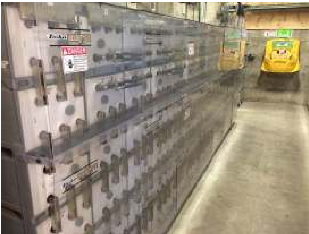
Figure 13. The National Park Service budgets, ideally, $100,000 per year for O&M of this PV energy storage system (308 kW PV; 1,920 kWh battery) on Alcatraz Island. Photo by Andy Walker, NREL
