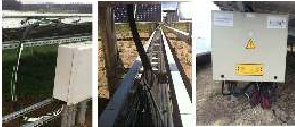
Figure 2. Maintenance of wire management systems depend on plastic wire ties and grommets, which can break or pinch wires (left); exposure to sunlight; wind and weight of ice (center); and access by chewing rodents (right). Photos by Andy Walker, NREL
