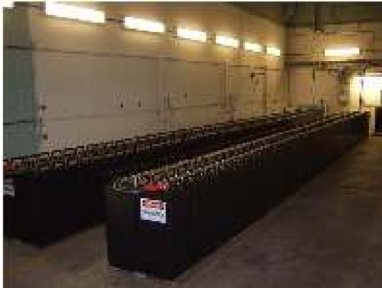
Figure 1. Two strings of batteries are recommended in design to allow O&M service of one string while the other string serves the purpose. Photo by Andy Walker, NREL
