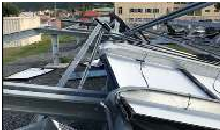
Figure 10. It might be the responsibility of the O&M provider to respond and ensure that storm damage is rendered safe both in terms of electrical hazards and loose components following an extreme weather event such as this damage in St. Croix in 2017. Photo by Andy Walker, NREL
