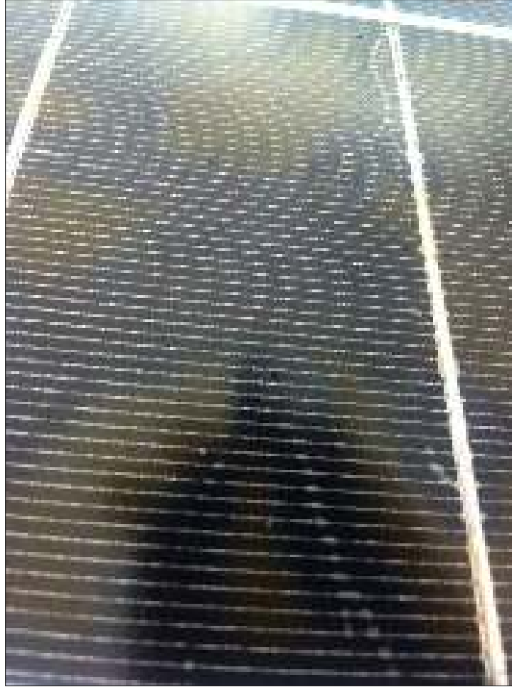
Figure 15. Snail trails in encapsulant are attributed to cracks in cells caused by flexure of the panel at the factory, shipping, or installation. The module would be covered by the performance warranty only if the cracks isolate fragments of the cell and reduce the output over time. Photo by Andy Walker, NREL
