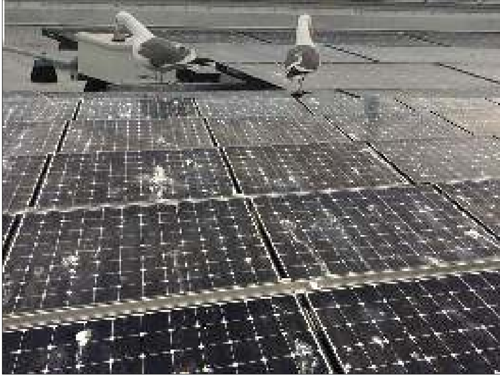
Figure 8. Bird populations are a source of soiling, as well as nests that need to be removed and seeds that can sprout on arrays. Photo by Andy Walker, NREL
