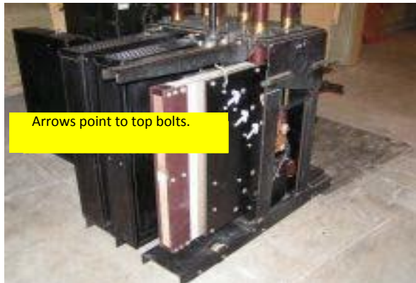
Figure 24 Top Bolts on an Arc Chute
