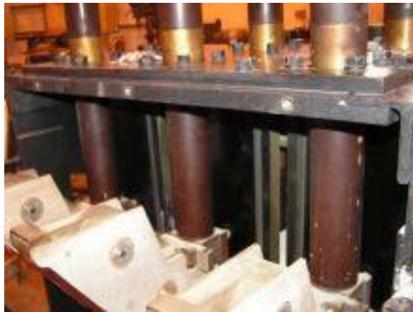
Figure 23. Load-Side Stabs and Separators
