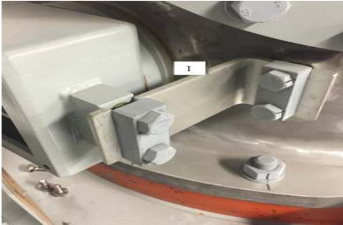
Figure 19. MEPPI Bonding Strap Arrangement
