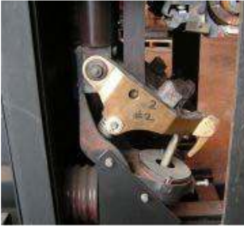
Figure 29. Installed Contact Assembly
