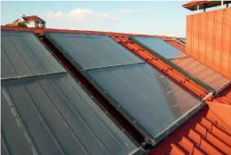
Figure 2.3 Photo of a solar hot water panel.
