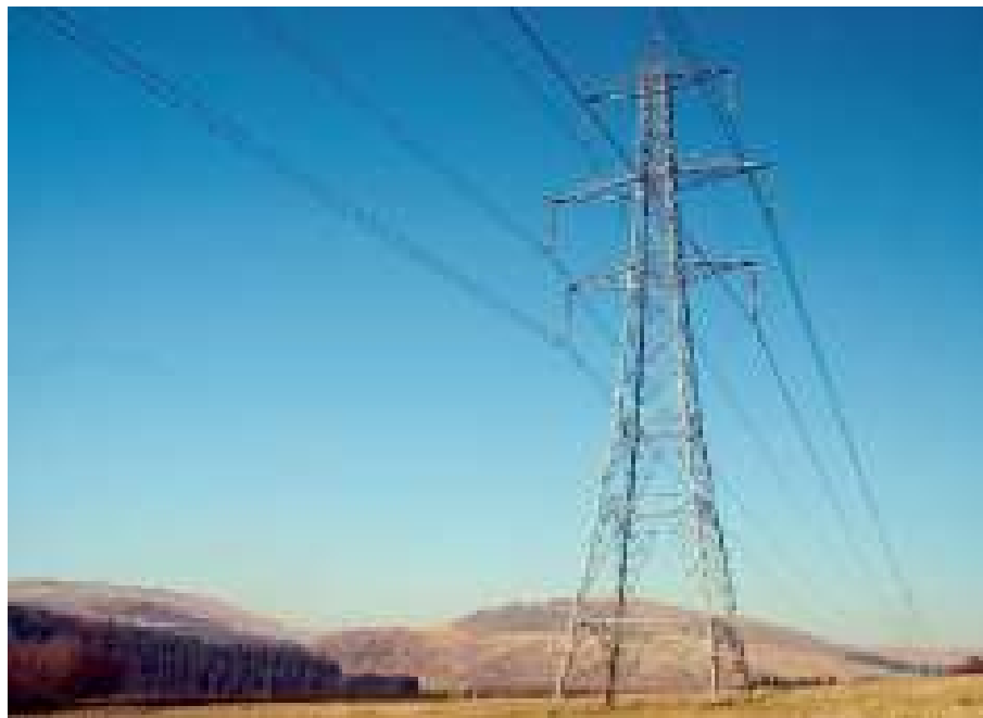
Figure 4.5 Transmission line steel pylon.
