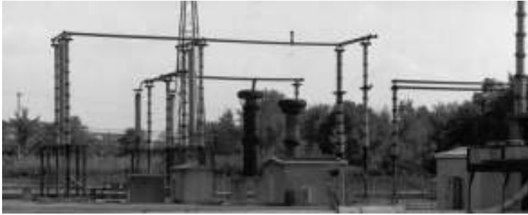
FIGURE 6.10 800-kV dc terminals of a converter station.
