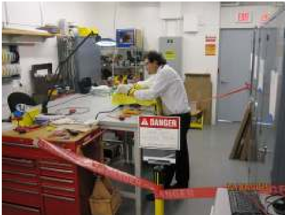
A DANGER barricade and sign indicating live testing and troubleshooting (MODE 2)
