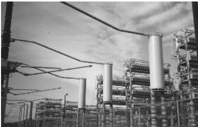
FIGURE 10.20 550 kV capacitor reactor.
