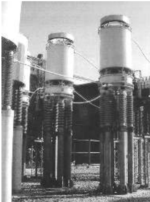
FIGURE 10.44 Tapped filter reactor with de-Q'ing rings.
