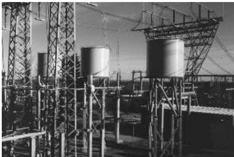
FIGURE 10.6 345 kV phase reactors.
