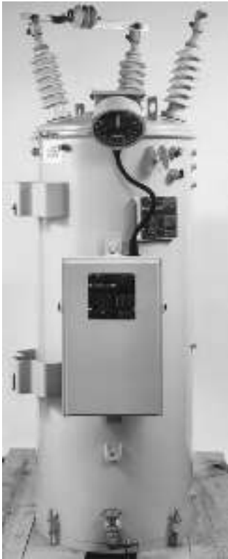
FIGURE 8.1 Single-phase step-voltage regulator.
