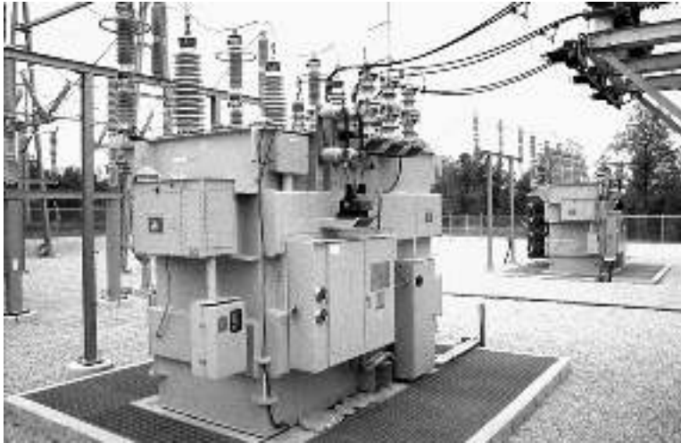
FIGURE 2.1 20 MVA, 161:26.4 \times 13.2 kV with LTC, three phase transformers.
