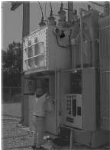
Externally mounted tap changer
