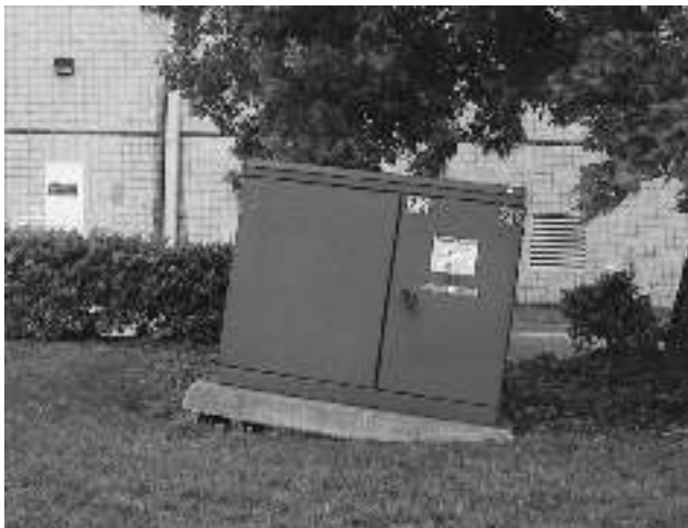
FIGURE 3.35 Tilting pad mount transformer.
