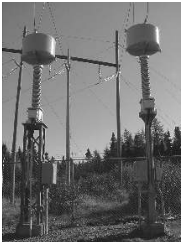
FIGURE 10.50 Line traps mounted on top of CCVTs.
