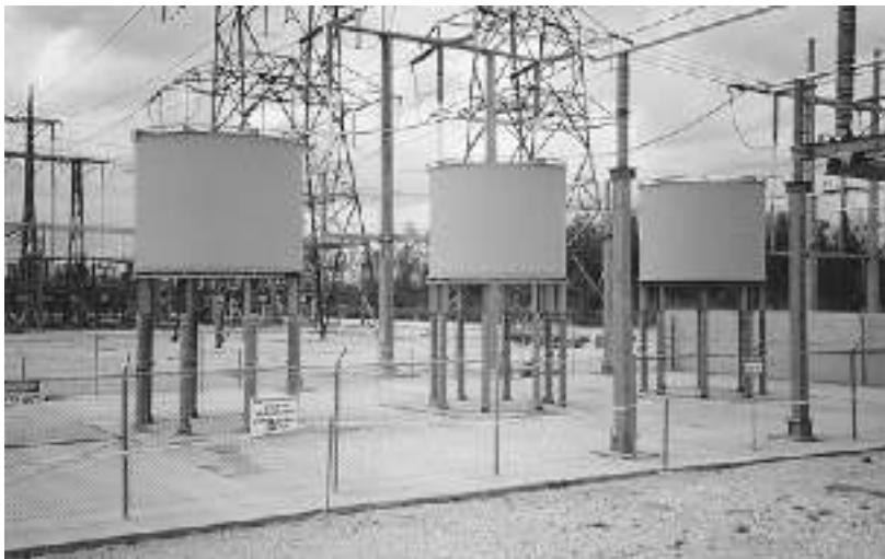
FIGURE 10.8 230 kV bus tie reactors.
