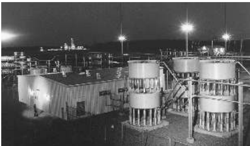
FIGURE 10.28 34 kV, 25 MVAR (per phase) thyristor controlled reactors.
