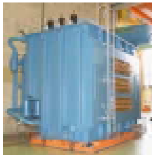
160 MVA steel EAF Transformer. Internal closure.
