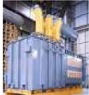
79 MVA Rectifier Transformer. Common tank.
