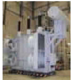
64 MVA Drives Converter Transformer. 12 pulse
