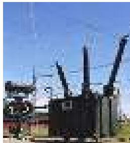
Shunt reactor, 400 kV, 150 MVar
