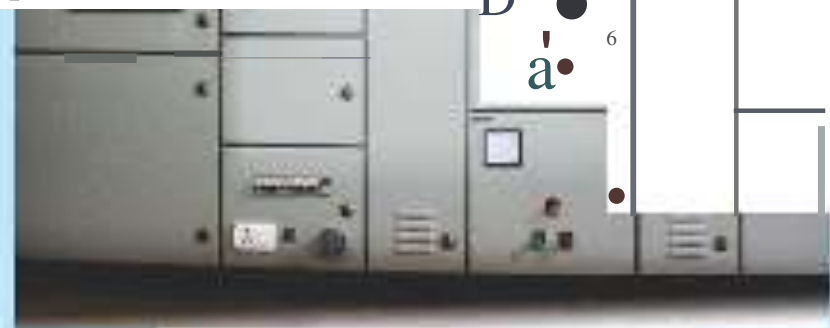
ACB- MCCB, MCC PANEL
