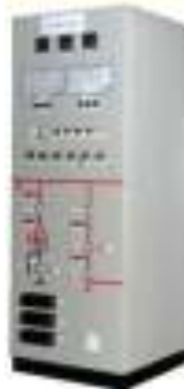
33 KV Relay Panel
