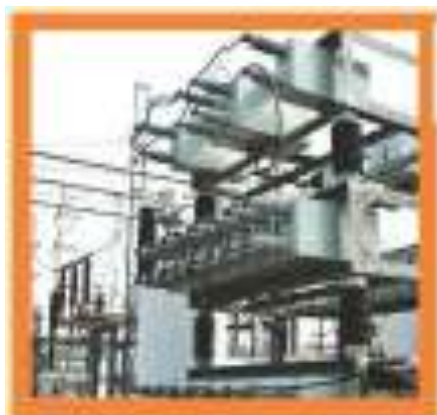
Open Rack Substation Bank
