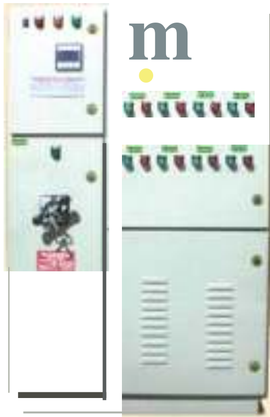
Capacitor Control Panel
