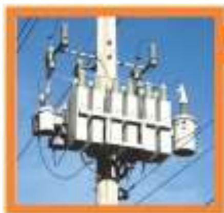
M.V. Pole Mounted Capacitor Banks
