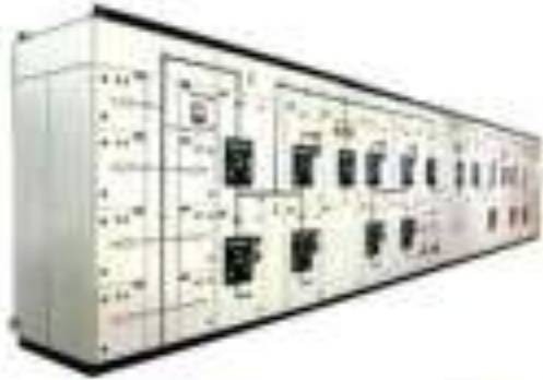
POC Control Panel
