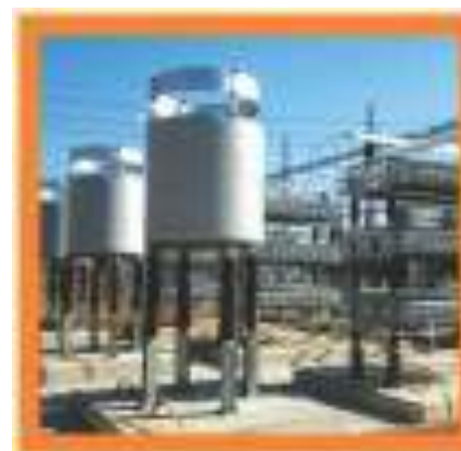
Harmonic Filter Bank
