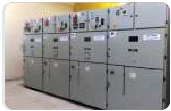
33kV VCB Panel
