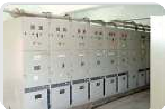
22kV VCB Panel
