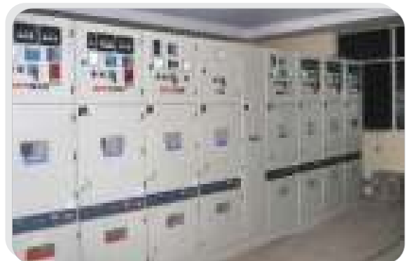
11kV VCB Panel
