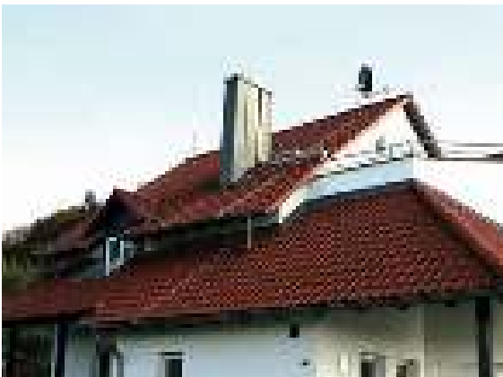
Figure 5.2.4.7 Protection of a residential building by means of DEHNcon-H (HVI light Conductor III)
