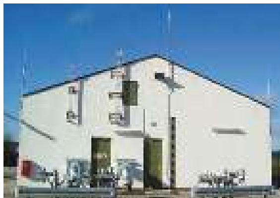
Figure 5.2.4.15 HVI Conductor installed on a gas pressure control and measurement system
