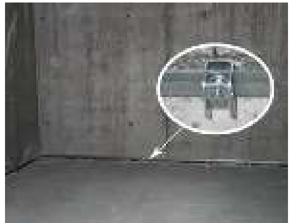
Figure 7.4.2 Ring equipotential bonding bar in a computer room
