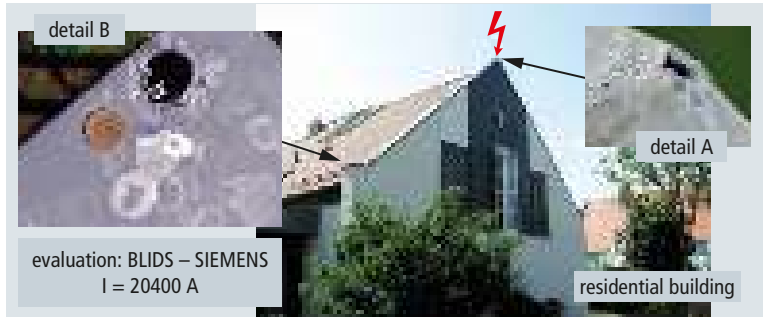
Figure 5.1.4.2 Example of damage: Sheet metal
