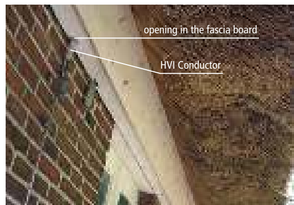
Figure 5.1.5.7 HVI Conductor led through the fascia board
