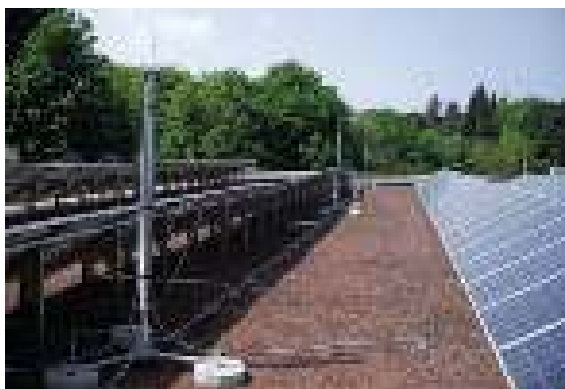
Figure 5.2.4.5 Protection of a PV system by means of a HVI light Conductor
