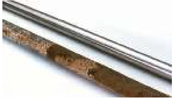
Figure 5.9.7 Corrosion of a galvanised earth rod (below) and a stainless steel earth electrode (above) after 2.5 years
