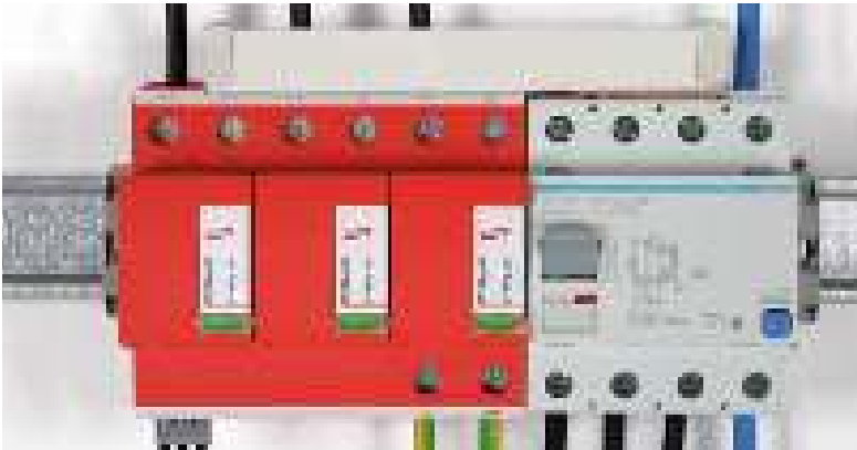
Figure 8.1.6.11 Series connection of the DEHNventil M TNC combined arrester by means of a busbar
