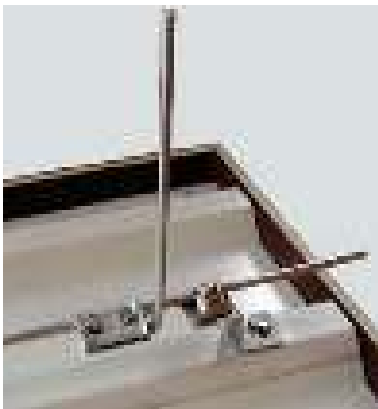
Figure 5.1.4.5 Sample construction of a trapezoidal sheet roof, conductor holder with clamping frame
