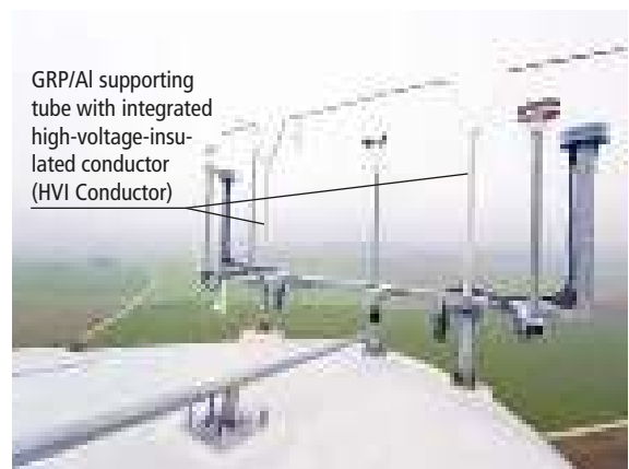
Figure 9.16.2 Example of an air-termination system for the weather station and the aircraft warning light
