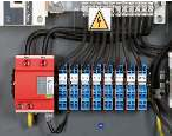
Figure 9.19.11 Surge protective device in a monitoring generator junction box
