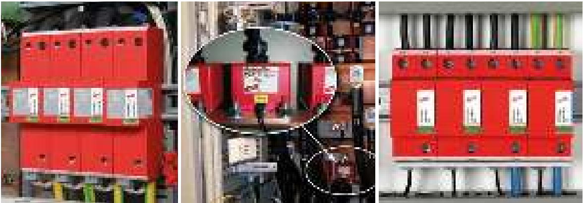
Figure 7.5.2.9 Lightning current arrester at the transition from LPZ 0 A to LPZ 1
