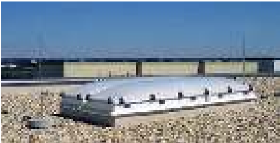
Figure 5.1.1.17 Protection of small-sized roof-mounted structures against direct lightning strikes by means of air-termination rods
