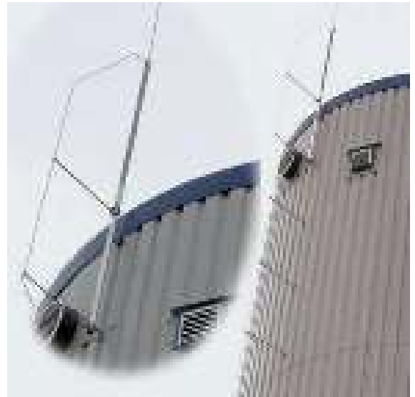
Figure 9.3.7 Protection of a fermenter made of metal sheets by means of an isolated air-termination system (source: Büro für Technik, Hösbach)
