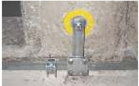
Figure 7.4.3 Connection of the ring equipotential bonding bar to the equipotential bonding network via a fixed earthing terminal
