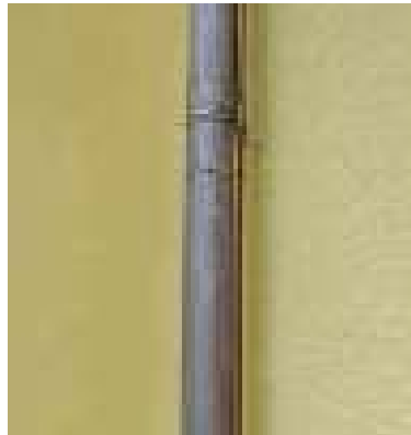
Figure 5.2.2.2.4 Down conductor installed along a downpipe
