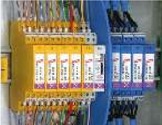
Figure 8.2.6.3 Monitoring of surge protective devices by means of the DRC MCM XT condition monitoring unit
