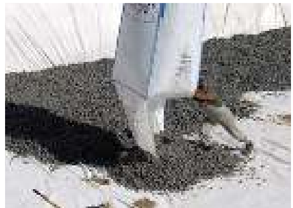
Figure 5.5.2.23 Perimeter insulation: Foam glass granulate is filled in; source: TECHNOpor Handels GmbH
