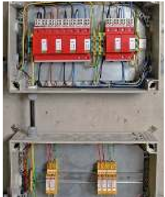
Figure 7.5.2.8 Lightning equipotential bonding for power supply and information technology systems situated centrally at one point
