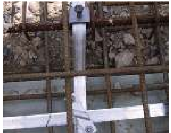
Figure 5.5.2.4 Foundation earth electrode in use
