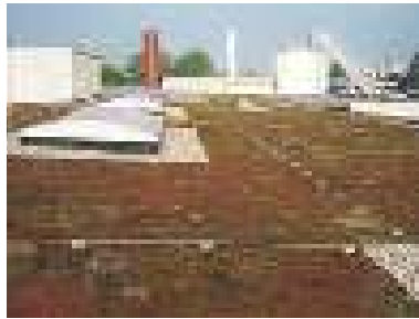
Figure 5.1.7.2 Air-termination system on a green roof
