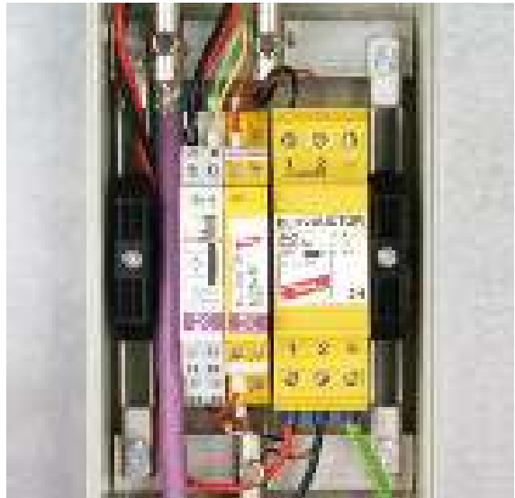
Figure 9.16.10 Protection of wind measurement equipment (anemometer)
