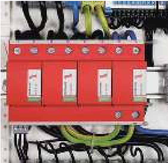
Figure 9.4.5 DEHNventil installed in a switchgear cabinet for protecting the power supply systems
