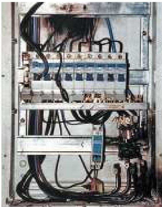
Figure 8.1.3.1 RCD destroyed by lightning impulse currents
