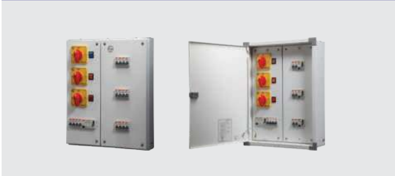
Metal DBs for Three Phase and Neutral (TPN ) supply distribution with selector switches for phase selection
