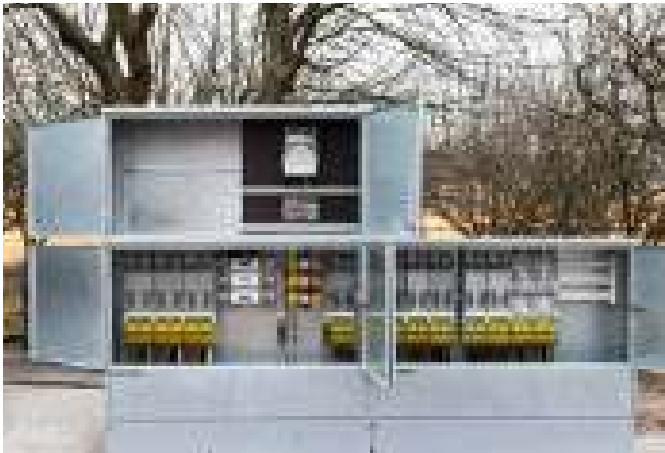
Cable distribution board, Sweden.
