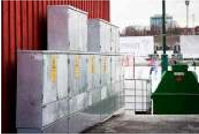
Cable distribution boards at Hedens bandy rink, Gothenburg, Sweden.
