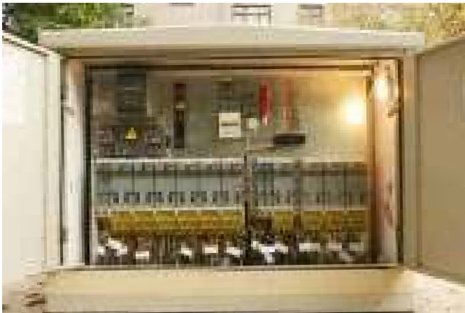
Kabeldon switching devices in a CSS, Latvia.
