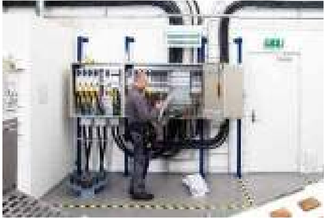
Distribution board in powder coated enclosure mounted on the wall in a switchgear room at a bakery, in Gothenburg, Sweden.
