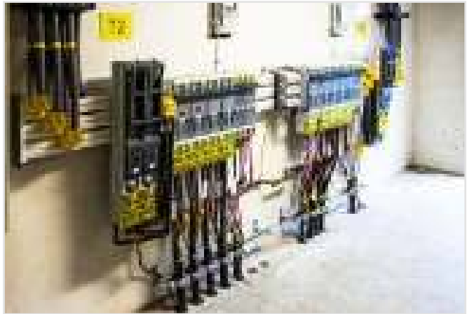
Examples of using Kabeldon products on the wall in low voltage switchgear, Sweden.
