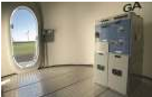
FBX-E in the mast of a wind tower, can be installed through a narrow door thanks to its compact size
