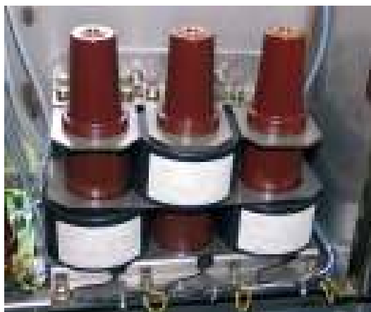
Bottom view of toroidal type current transformers on external-cone cable plug-in terminals (T2 Function)
