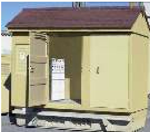
FBX-C in a MV/LV substation – chosen for its compact size
