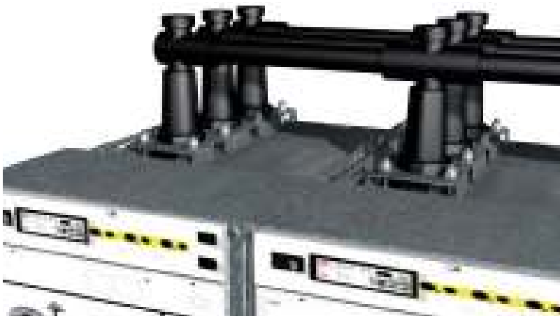
View of the busbars
