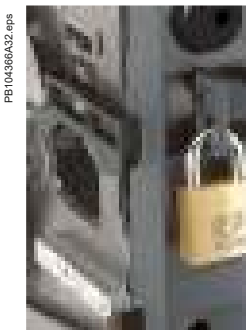
"Disconnected" position locking by padlocks.
