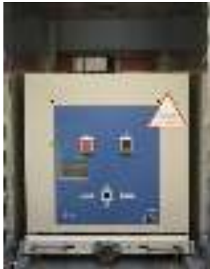
CB in Test Position
