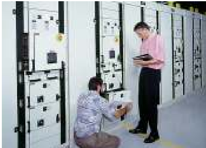
Motor Control Centre (MCC).
