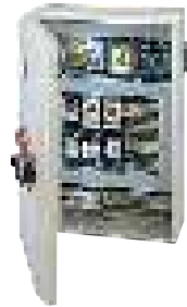
Automatic control panel or machine panel.
