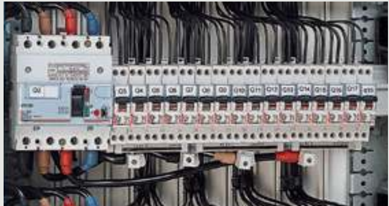
Row of single phase outputs supplied via a DPX 125 (100 A)
