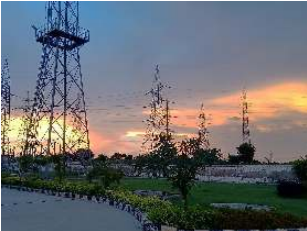
Figure 32. Lattice steel structures of overhead power lines
