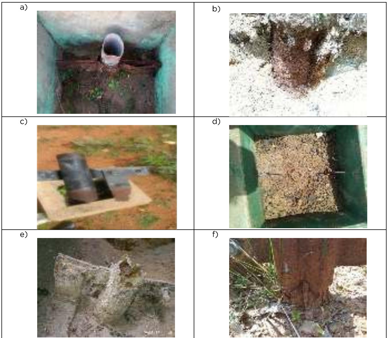
Figure 21. Corroded earth electrodes
