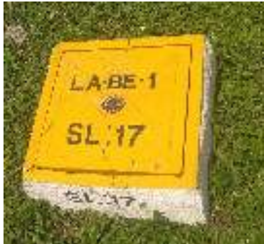
Figure 19. Earth pit with proper maintenance
