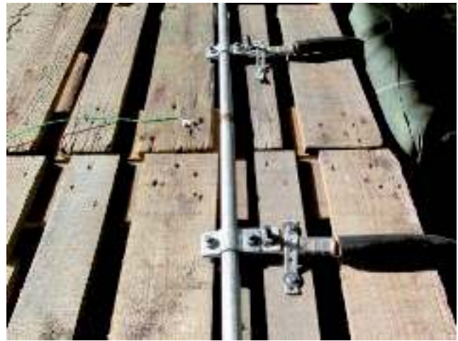
Short-circuit current test on earth rod
