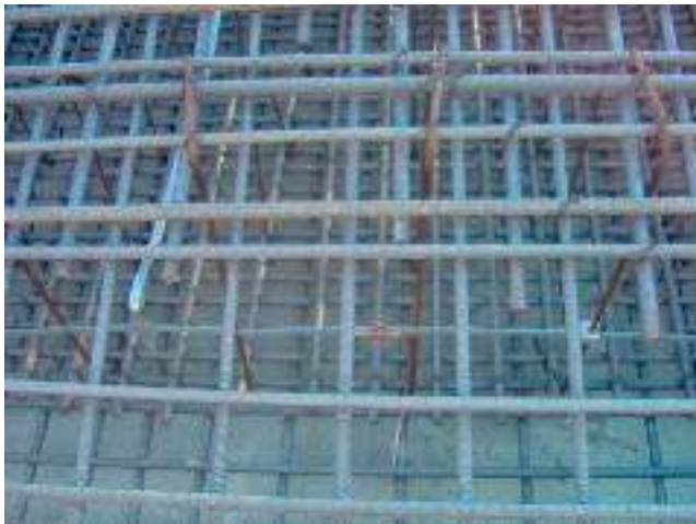
Earthing system of a wind power plant
