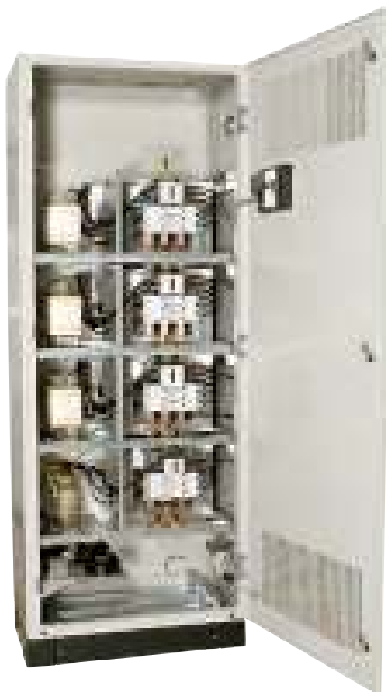
< Alpmatic step capacitor bank
