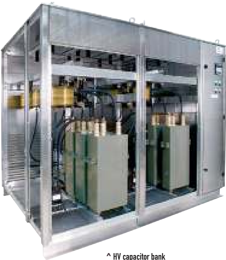
^ HV capacitor bank
