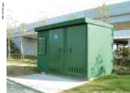
(a) Ground level walk in type substation
