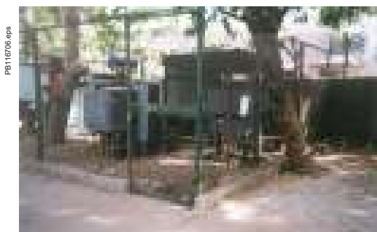
Fig. B53 Outdoor substation without enclosure
