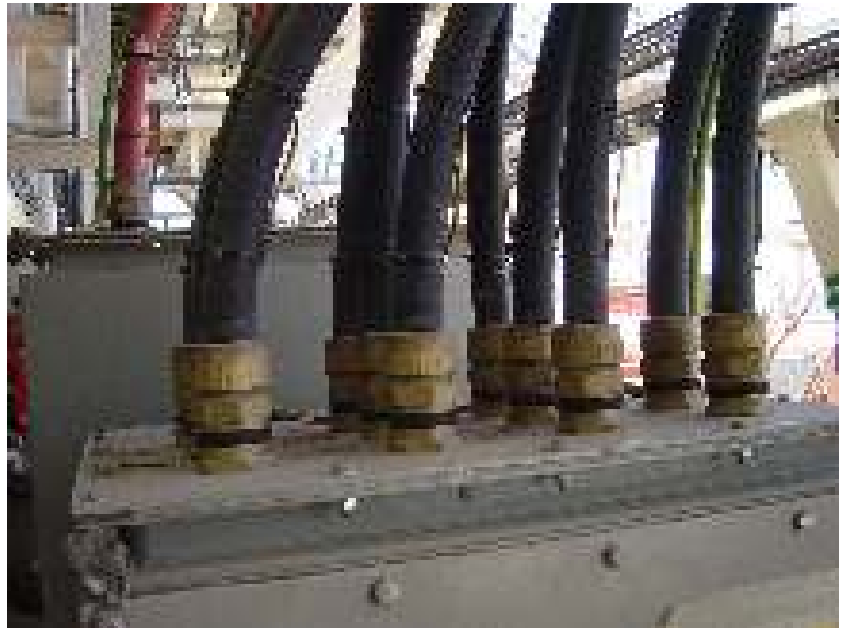
Figure 207: Flameproof cable glands installed on an enclosure
