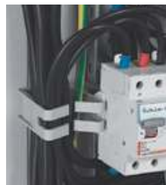
^ The enclosures have wiring guide rings
