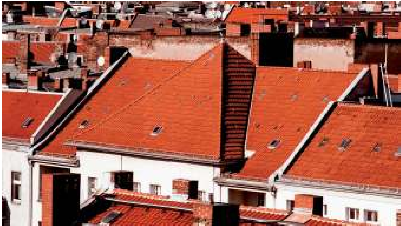
Firewalls prevent the spread of fire
