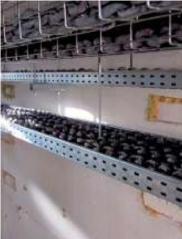
Cable tray with high mechanical load before...
