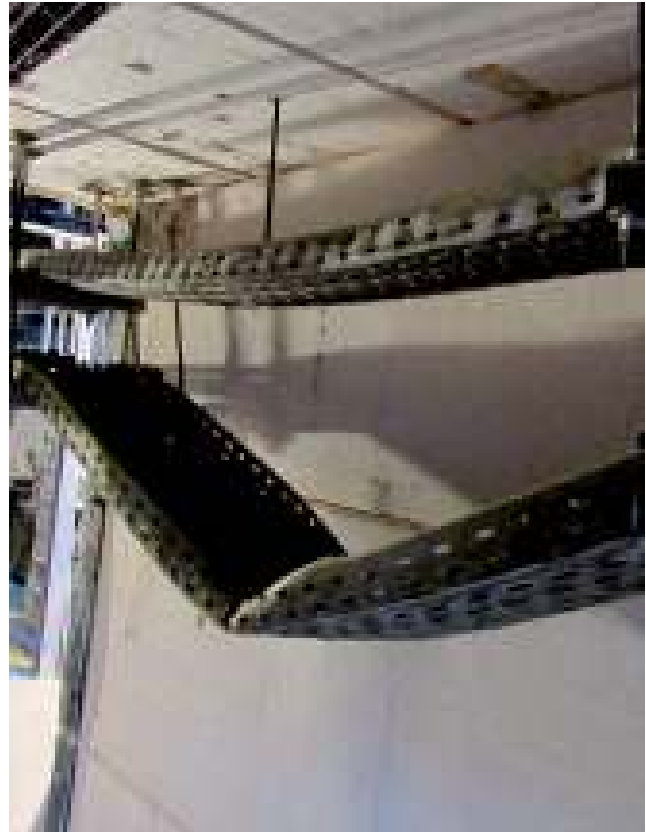
...and after fire testing
