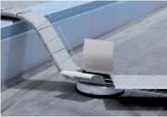
Bandaged cables routed over a firewall
