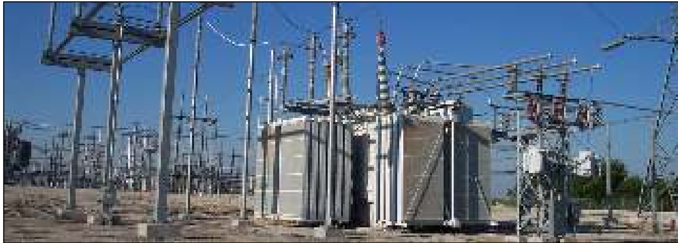
Relative Size of HV and EHV Power Transformers
