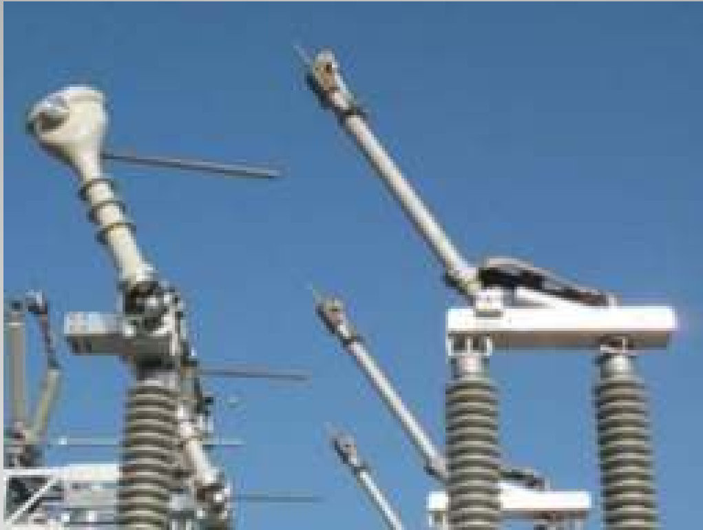
Load and Line Switcher
