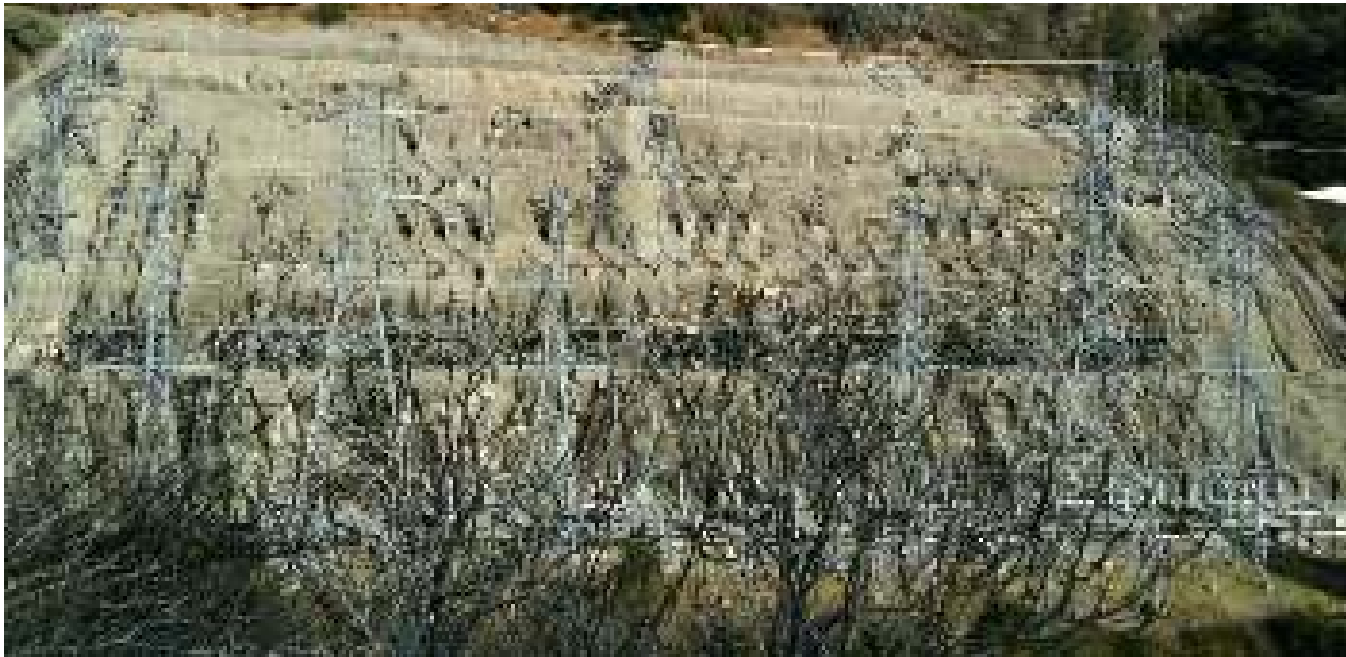
230 kV Generating Substation – Built on the side of a mountain
