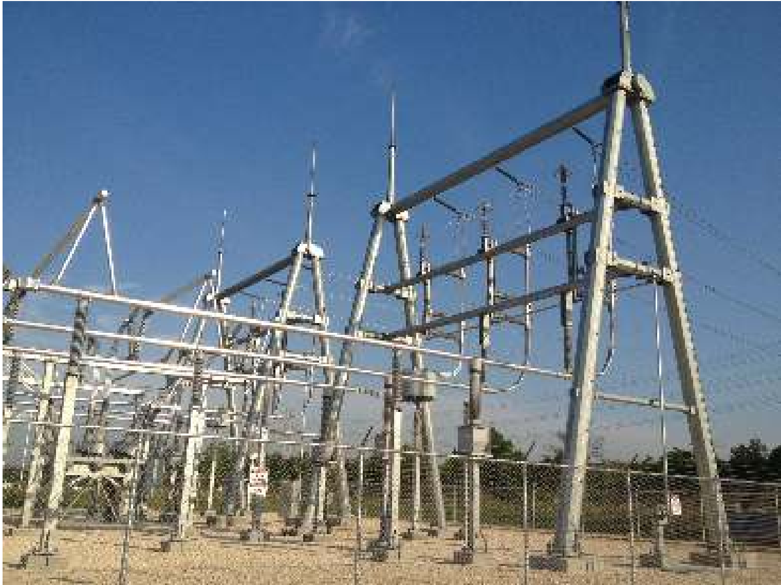
Typical 138 kV Substation
