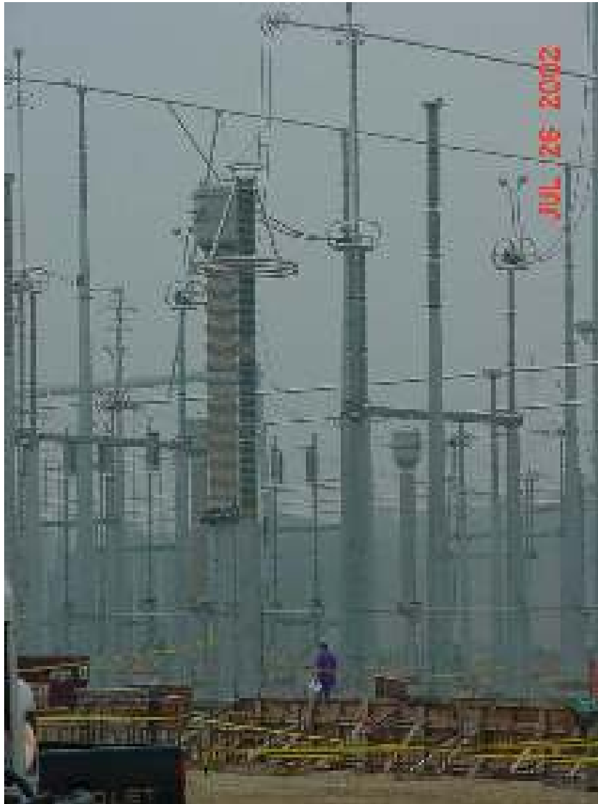
765 kV Generating Substation
