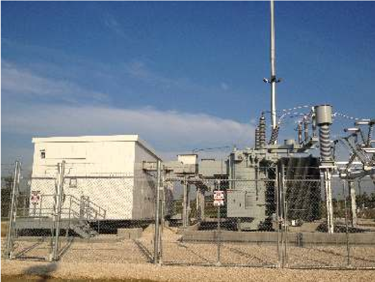
Typical 138 kV Substation
