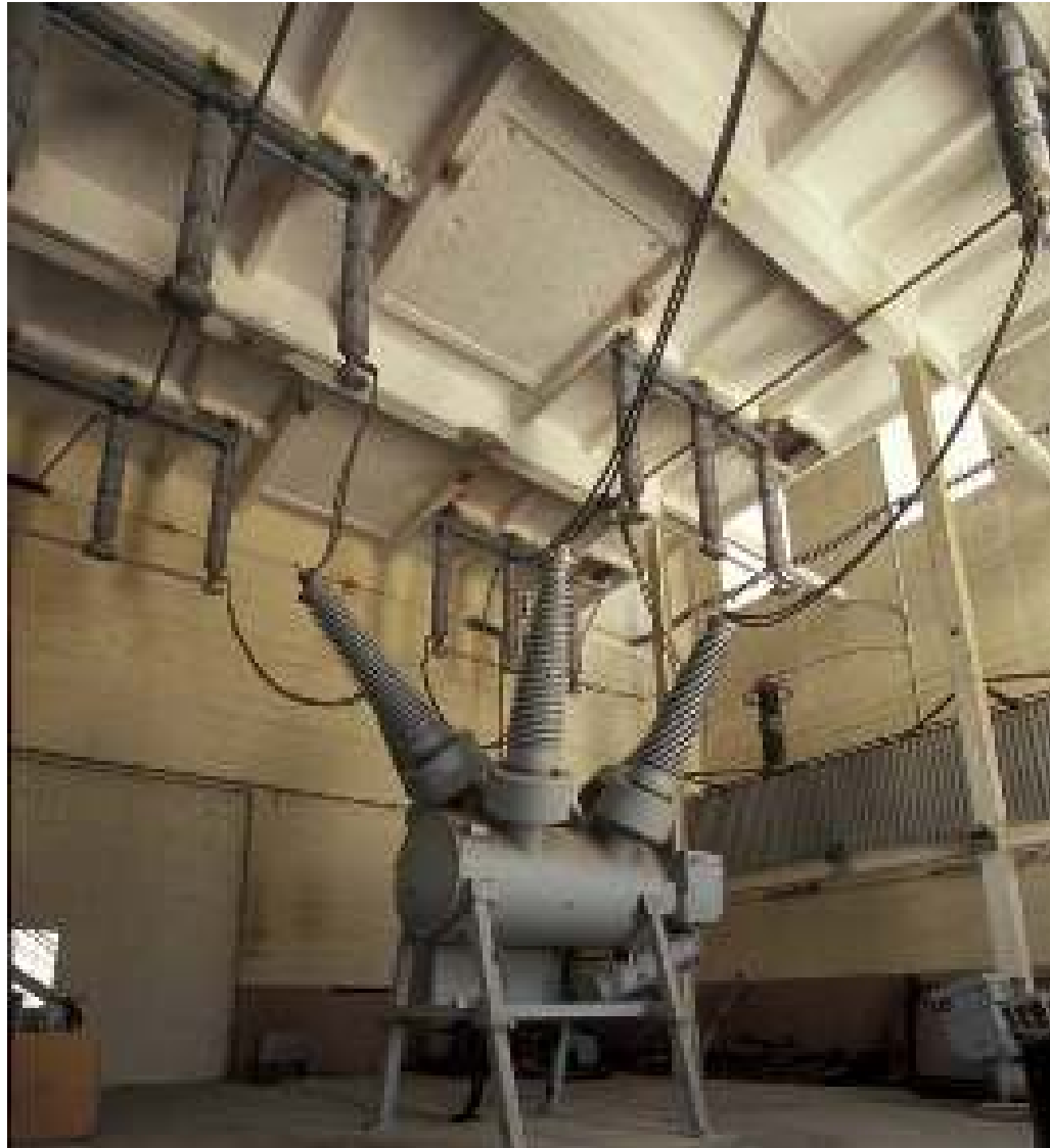
230 kV Indoor Generating Substation
