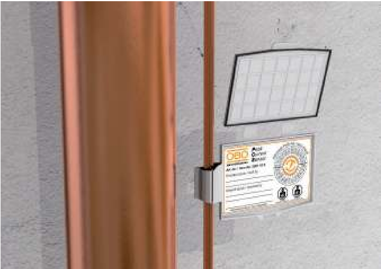
PCS sensor on a down-conductor
