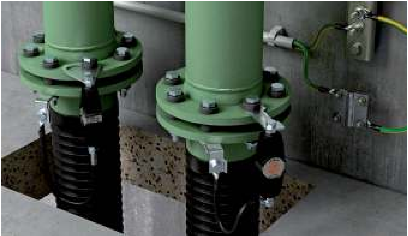
Spark gap mounted on insulating sections
