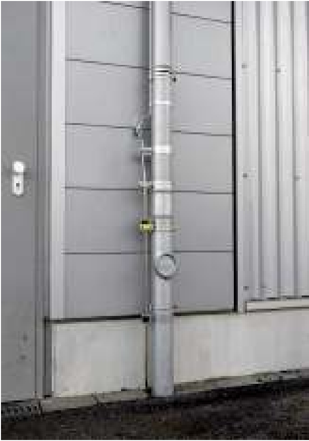
Lightning down-conductor at a downpipe
