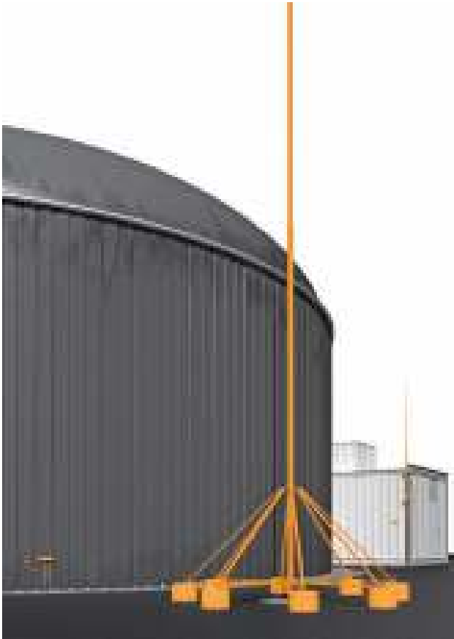
Tele rods at biogas plant
