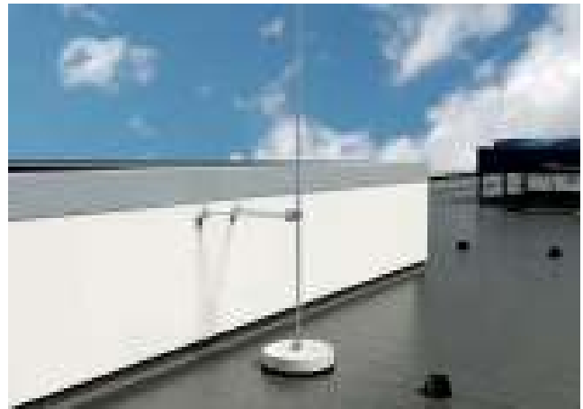
Isolated lightning protection with insulating beams
