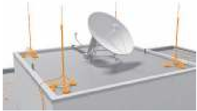
Isolated lightning protection with air-termination rods
