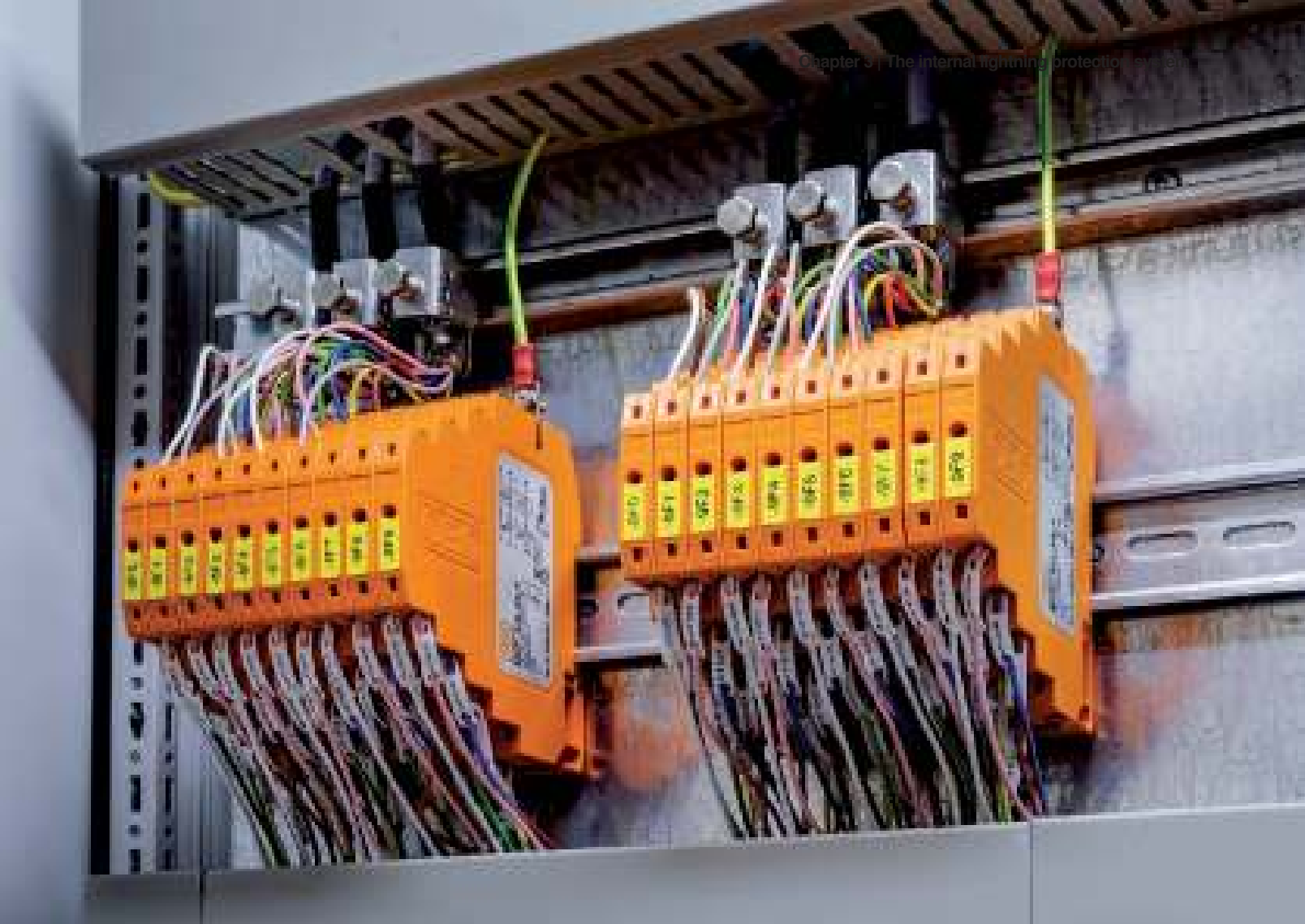
MDP lightning barriers in an switching cabinet
