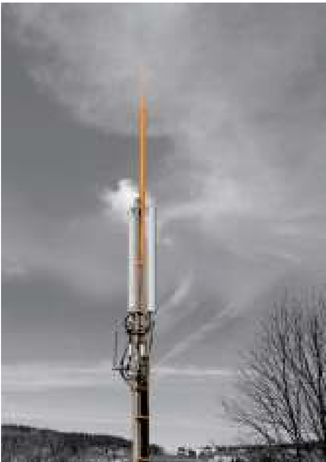
Cell tower with isCon® conductor
