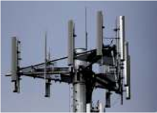
Mobile telecommunications mast
