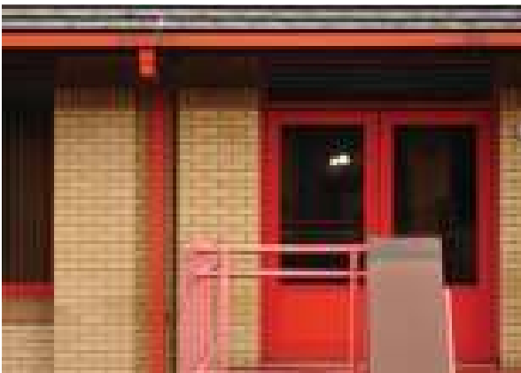
Figure 54. Example of poorly located a down-conductor.
