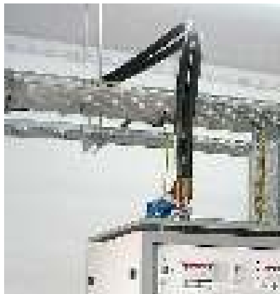
Figure 113. Incoming antenna circuits require protection.
