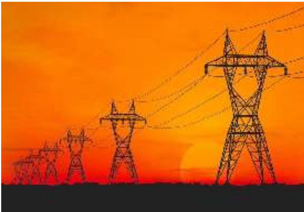
Figure 45. Ground wires in transmission lines
