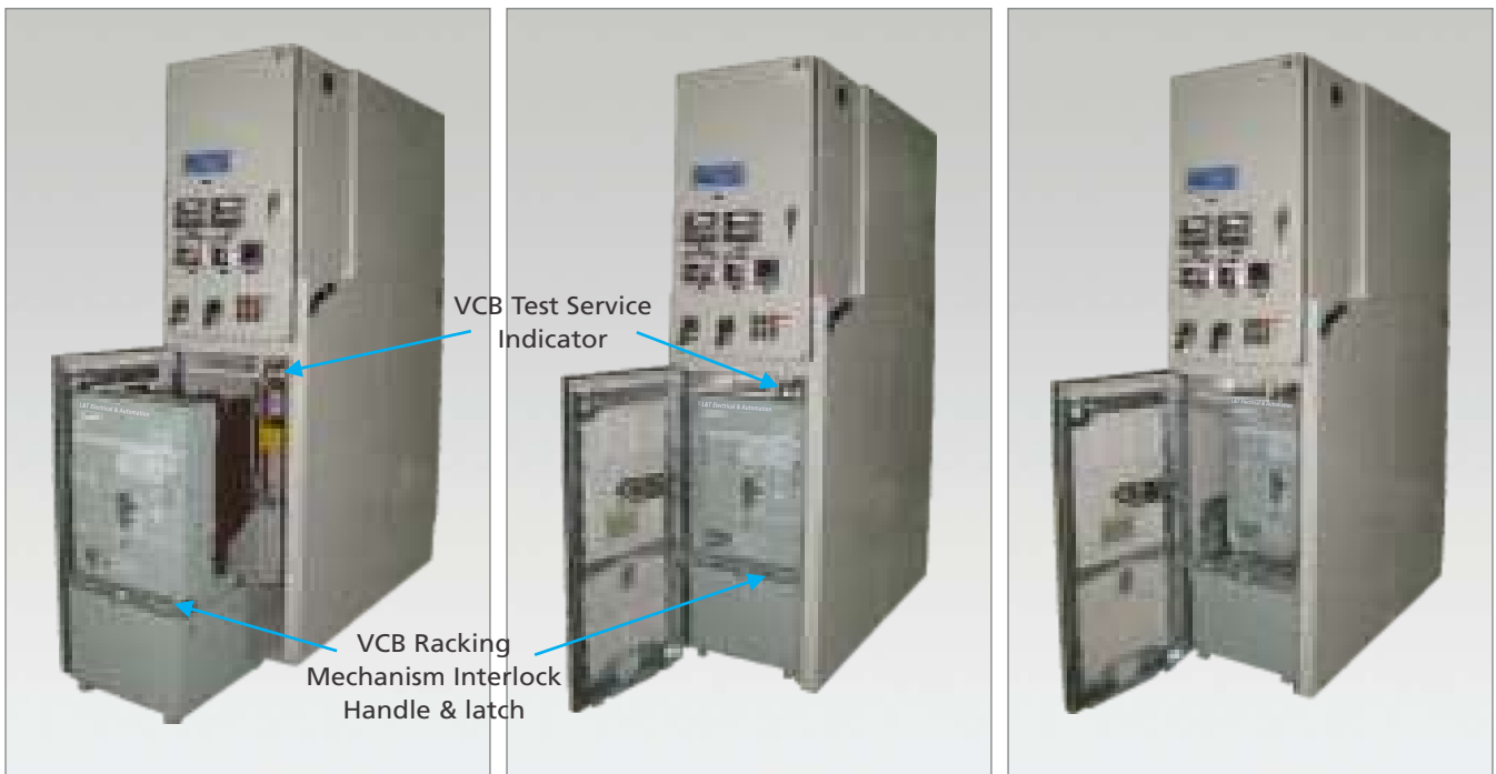
Figure 5.1 A - VCB in Disconnected
