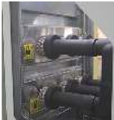
Isolated / test position
