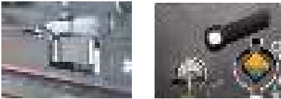
CB in isolated/test position - earthing switch OFF and shutter open
