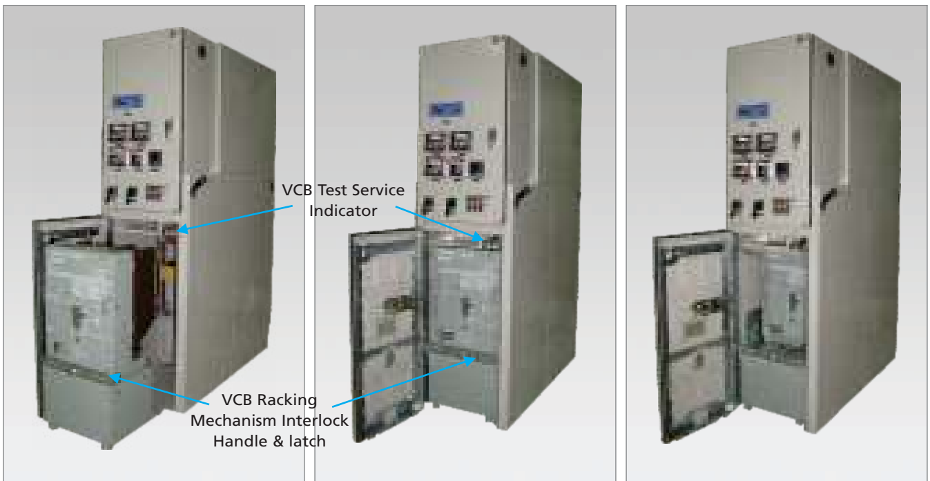
Figure 5.1 A - VCB in Disconnected
