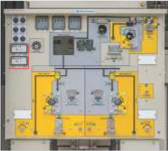
Figure 3.7.4: Fault Passage Indicators
