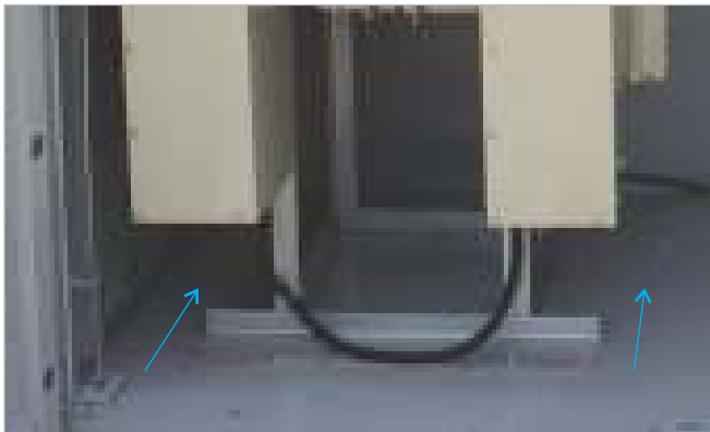
Figure 5.5.1 - HT cable gland location at RMU
