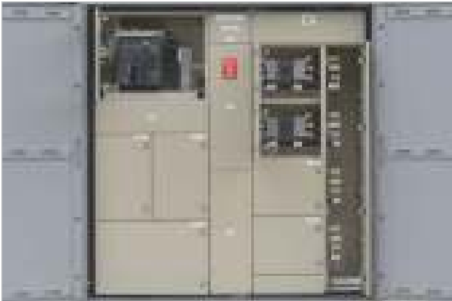
Figure 3.5: Low Voltage Compartment
