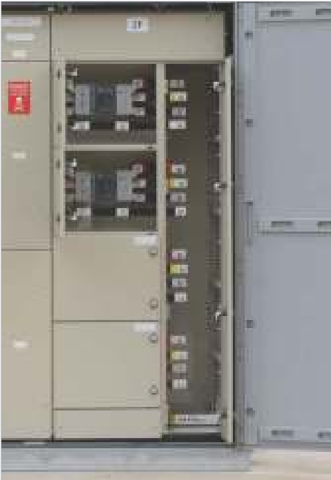
Figure 6.4.3 - LT Panel Cable Termination
