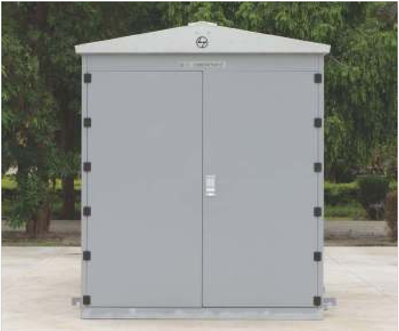
Figure 1: Compact Secondary Substation
