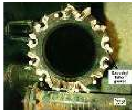
Figure 7.3.7. Failed gasket on blind flange.
