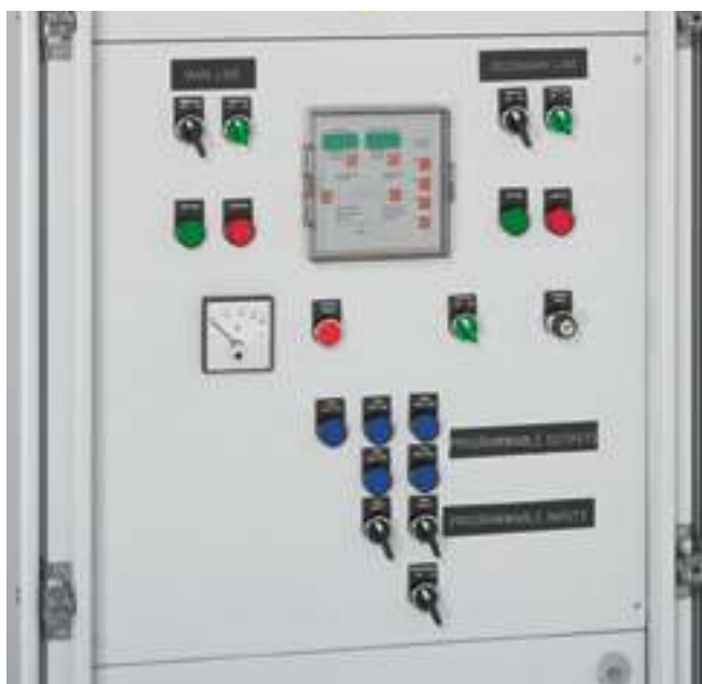
Supply inverter > control panel with control unit
