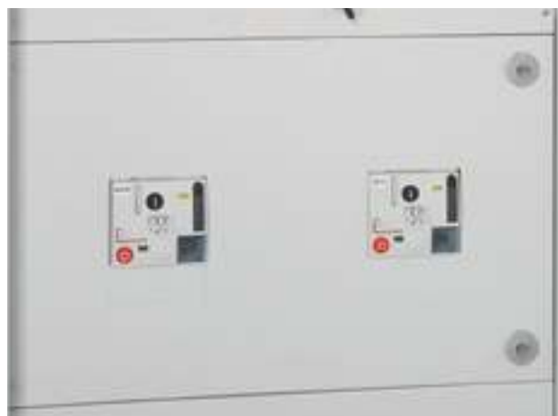
^ DPX supply inverter with motor-driven controls
