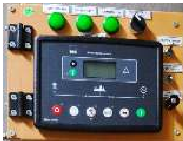
Fig. C4.4 Typical Engine Control Panel
