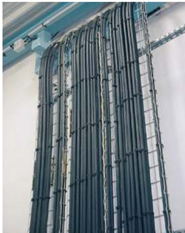
^ A neat cable layout is essential with regard to the fire risk
