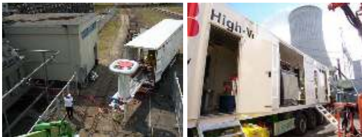
Figure 4.6 - Examples of AC tests on-site
