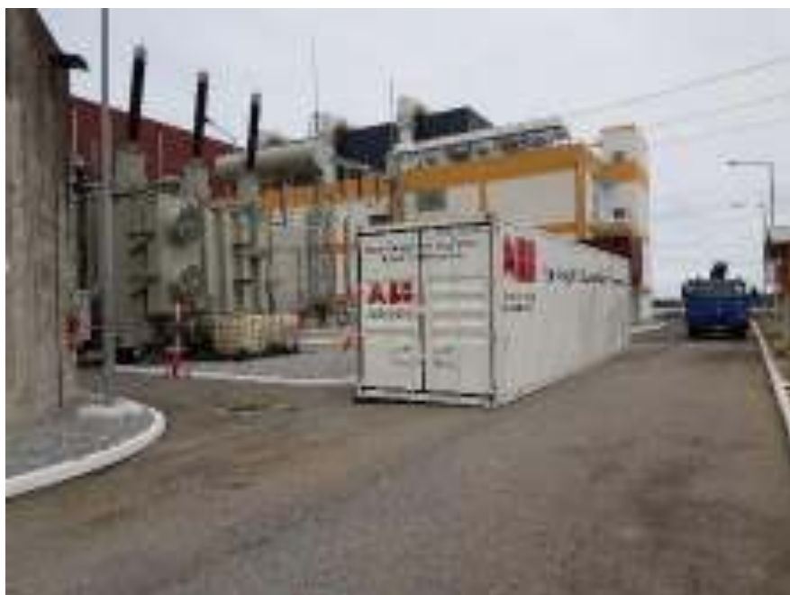
Figure 4.24 - AC mobile test system used for applied and induced voltage test
