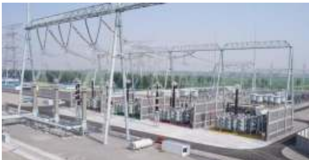
Figure 2.52 - UHV AC on-site assembly transformer in service (spare phase on the right side)
