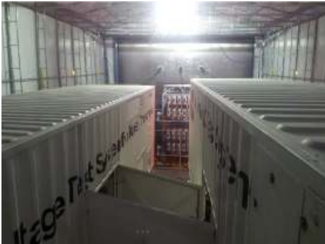
Figure 4.27 - Two AC mobile test systems used for temperature-rise test shown in front of the compensation unit
