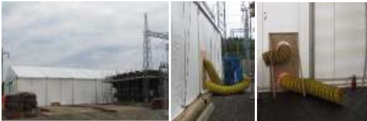
Figure 3.11 - Temporary Building Next to the Transformer Pad with Air Control
