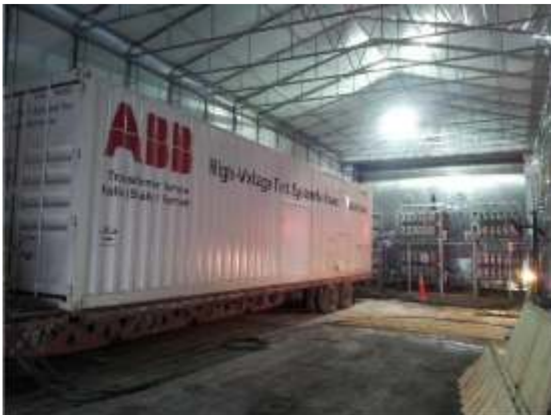
Figure 4.26 - AC mobile test system used for temperature-rise test shown in front of the compensation unit
