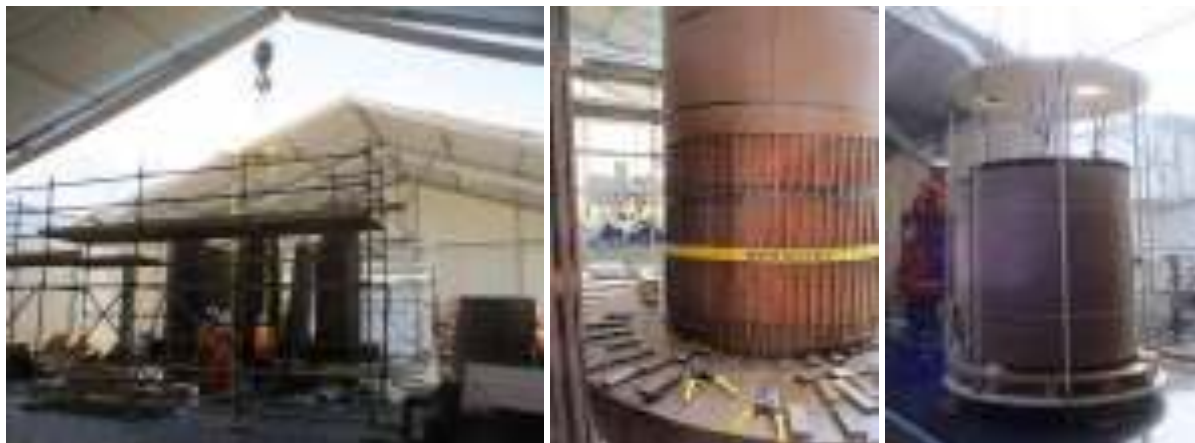
Figure 3.13 - Windings Being Removed from the Core/Windings and New Windings
