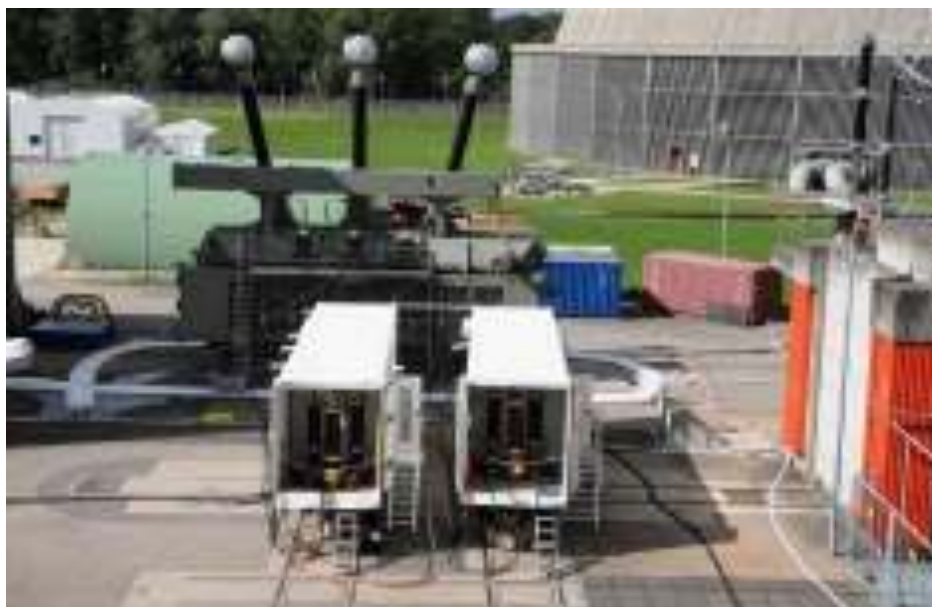
Figure 4.10 - AC test with 2 mobile test systems in parallel
