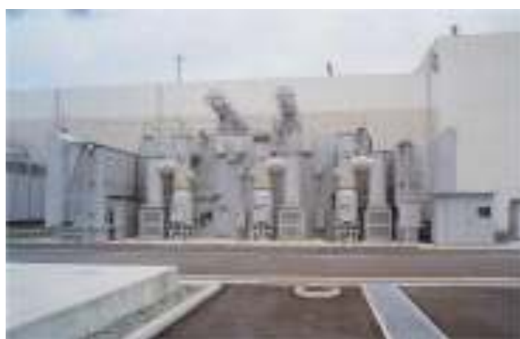
(a) Case 1 - 872 MVA, Core-form converter transformer
