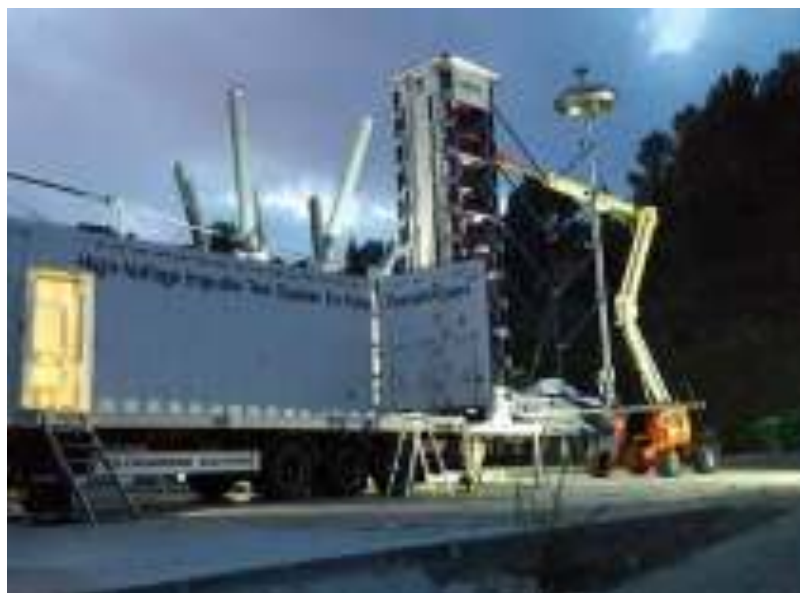
Figure 4.20 - LI impulse generator
