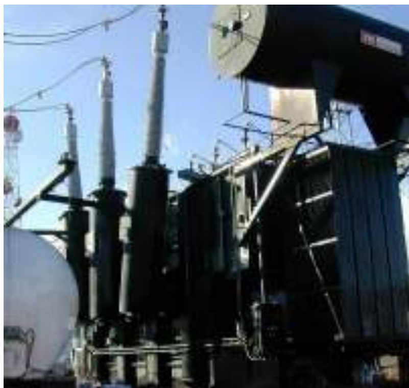
Figure 3.10 - Original transformer in service prior to the failure
