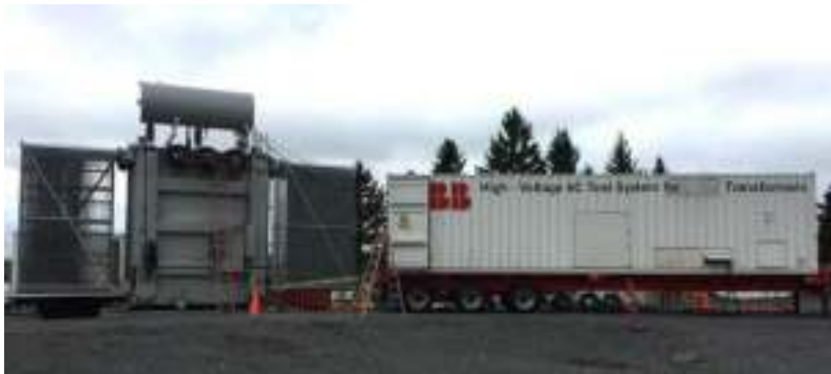
Figure 3.9 - Assembled Transformer Undergoing Final HV Field Induced Voltage Test
