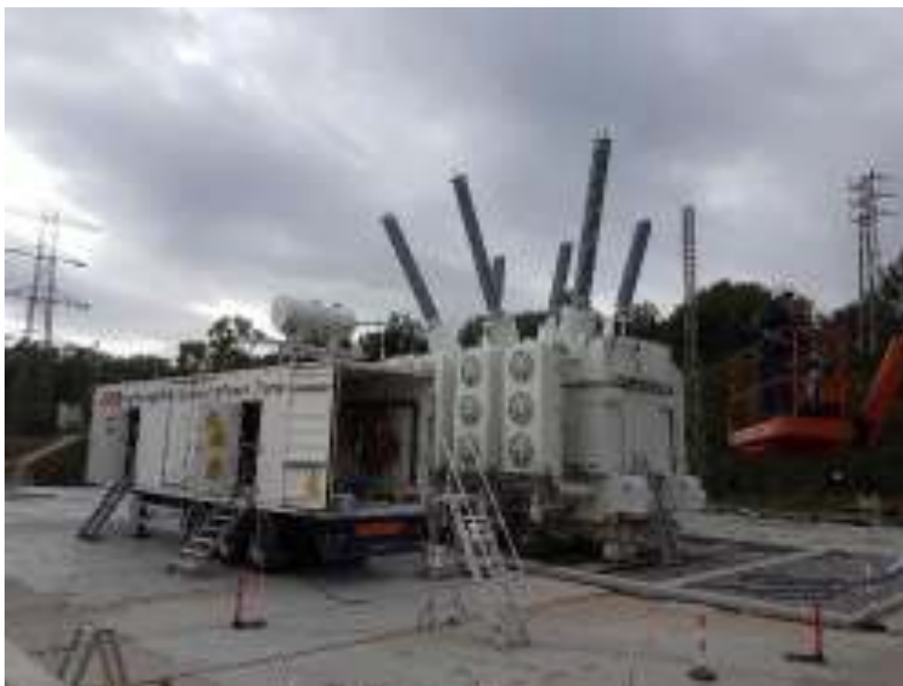
Figure 4.21 - Mobile test system used for applied and induced voltage test
