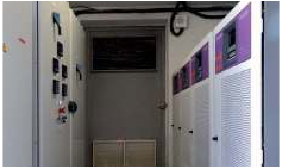
Energy storage facility at the Carros HVA/LV substation.
