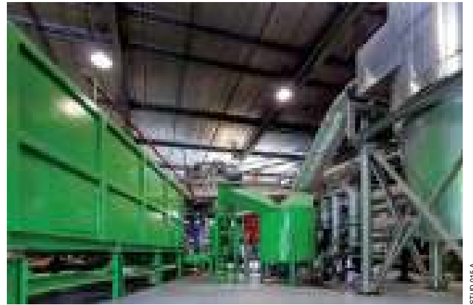
Cogeneration plant connected to an ORC (green mini power plant)
