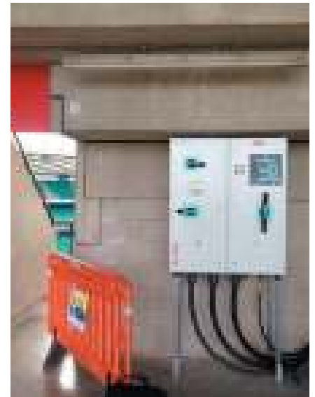
ATyS Bypass double line 250 A integrated in the stadium installation
