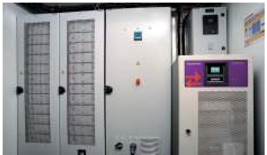
Left to right: battery storage cabinet, distribution panel and the Sunsys PCS 2 converter.
