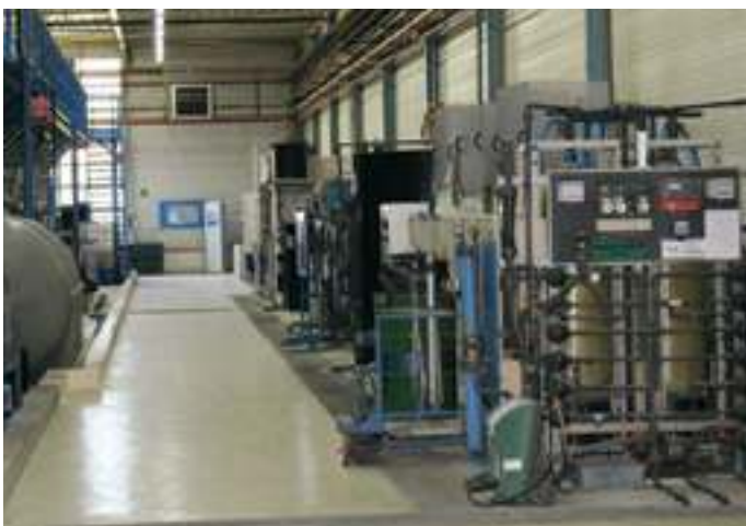
< Legrand has been involved in the reduction of the environmental impacts of its sites for many years, as in the Altis production plant: paint effluent treatment plant
