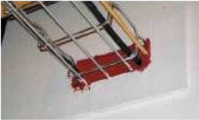
Filling of a fire barrier partition feedthrough with plaster and intumescent paste
