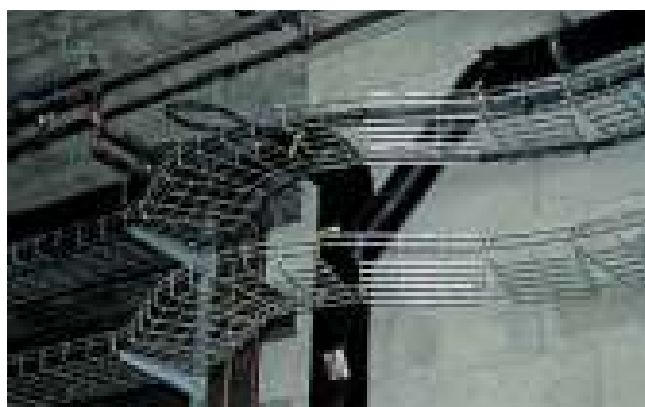
^ The configuration of the site, obstructions, the co-existence of different networks sometimes lead to complex routing
