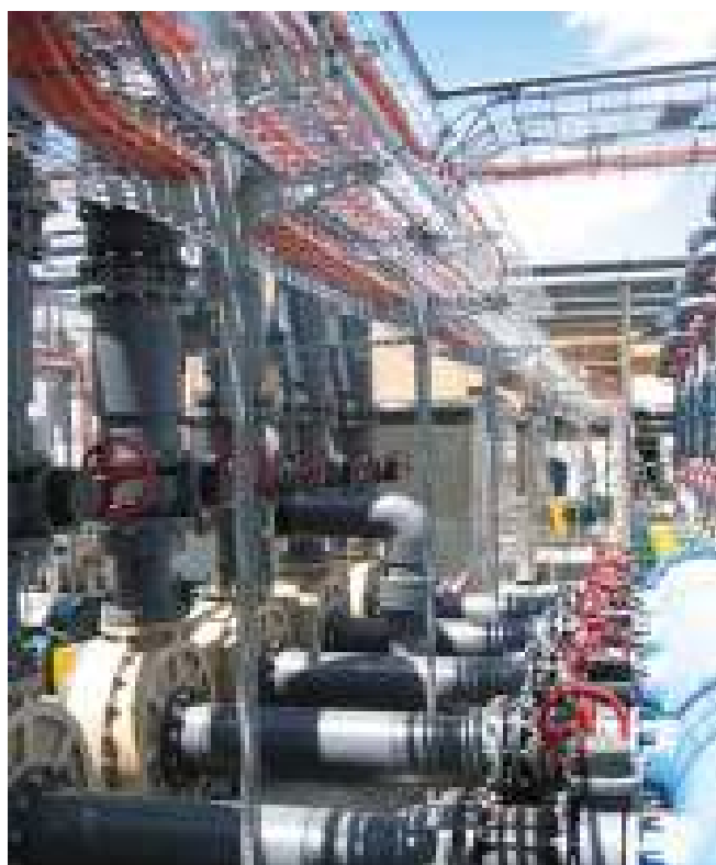
Wire cable trays used outside in this oil installation supporting cables chosen for their suitability for outside conditions
