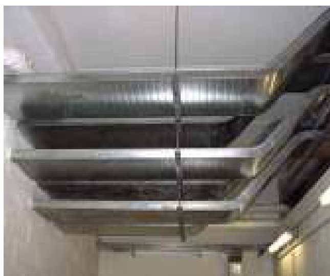
^ Metal cable trays with wall feedthroughs
