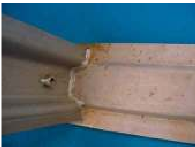
Traces of corrosion on the stainless steel consoles caused by discharges of iron particles due to grinding or machining assumed to be nearby. A risk that may have unacceptable aesthetic consequences...
