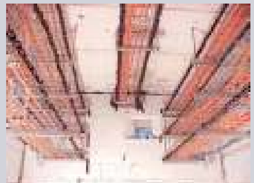
Cablofil cable trays inside the oven before the test
