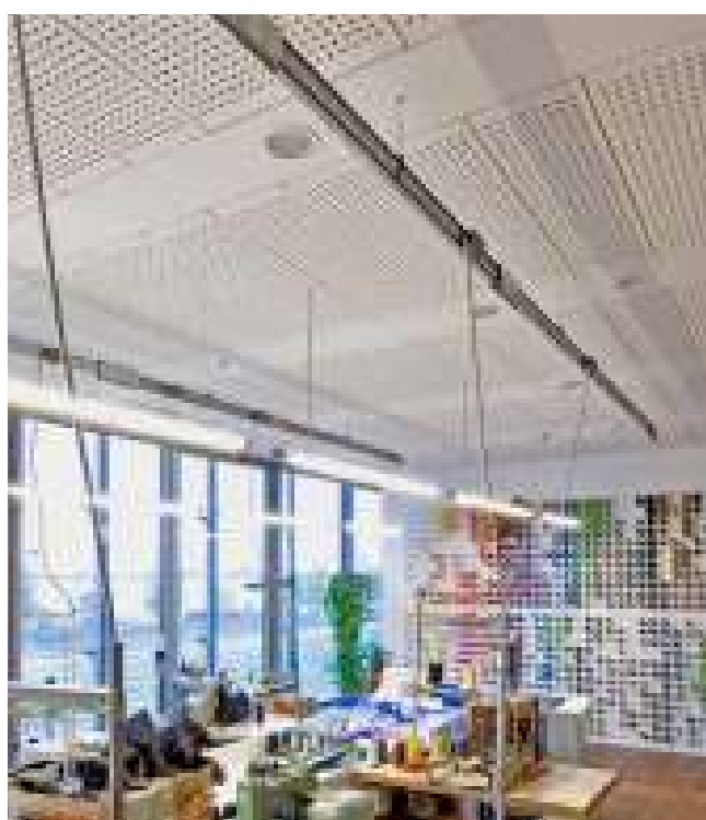
^ Legrand LB low power prefabricated busbar systems in a sewing workshop
