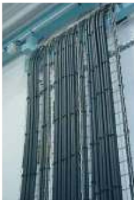
Careful layout of the cables complying with both the grouping rules and the precautions against fire
