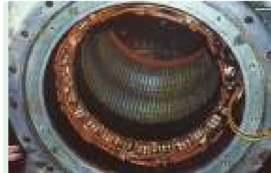
Stator of synchronous motor
