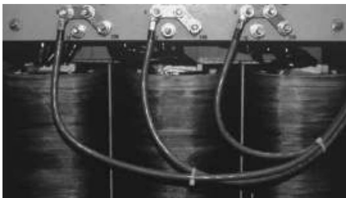
Figure 4.24 A medium-power, three-phase transformer.
